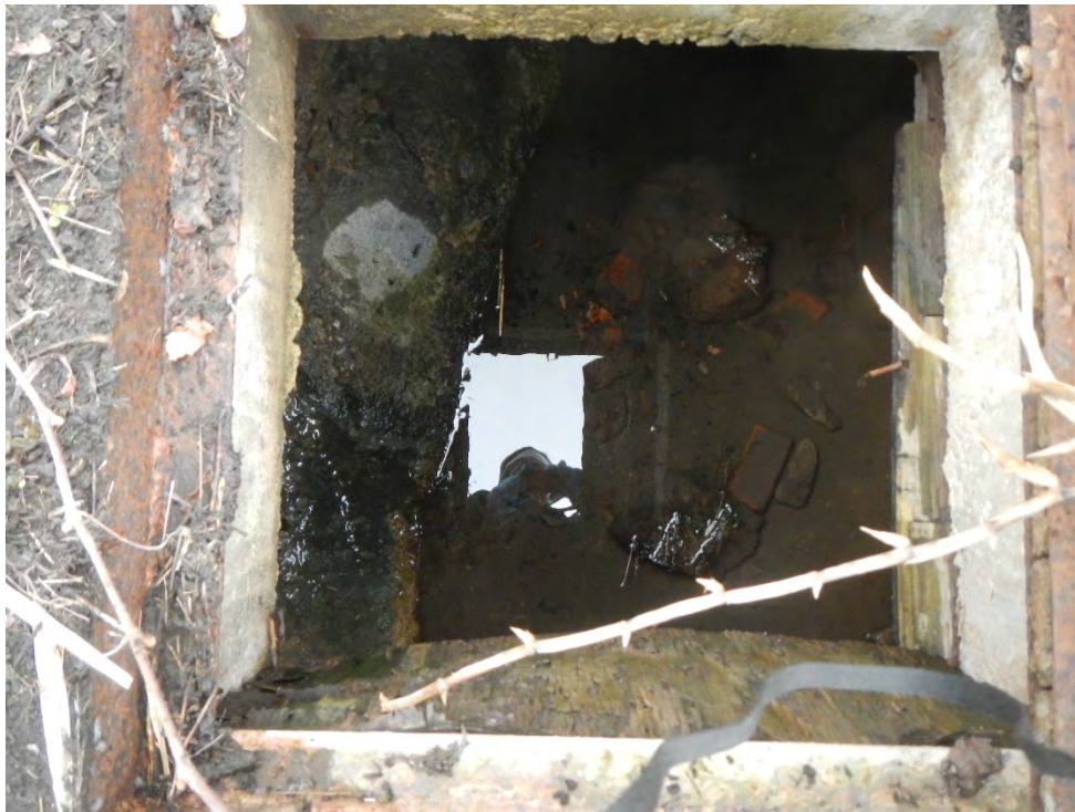
Photo 27 - View of interior of MH A-9 east of Site
