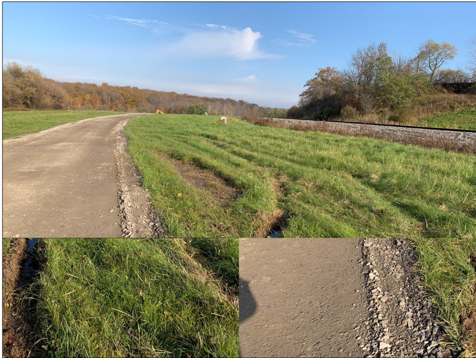
Photo 2 Site facing north along access road. Ruts shown from vehicle pulling off road
