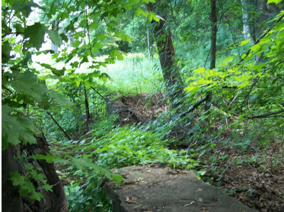
Figure 9-11. Photograph of the historic raceway wall shown in Figures 9-9 and 9-10, and the third spillway (center) on the Dussault property. View looking east. Photograph taken by Glenn May on July 14, 2008.
