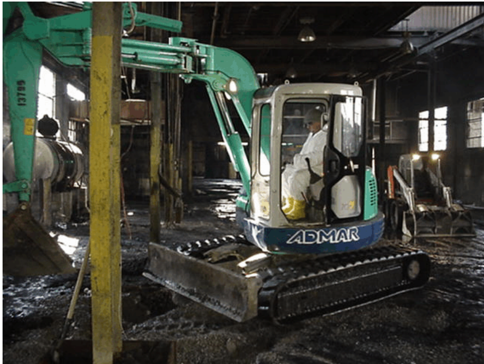
Figure 4-11. Photograph of the debris stockpiling operation at the Dussault Foundry Site. Photograph taken by Brian Sadowski on April 10, 2003.
