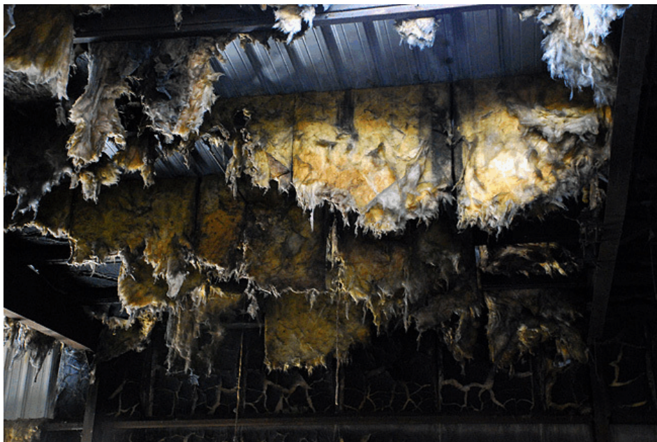
Figure 3-8. Photograph of the dilapidated buildings of the Dussault Foundry Site. Exact location is unknown. Photograph from the Urban Exploration Resource website at www.uer.ca .
