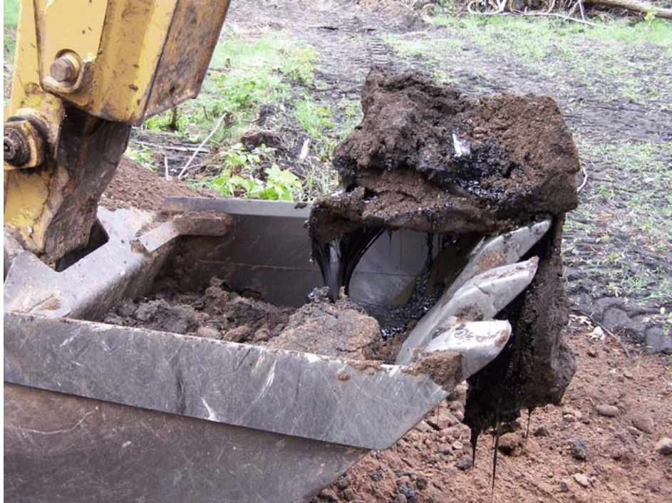
Figure 6-5. Photograph of the drum excavated from test pit SUB-90 that contained a tar-like waste. Photograph taken by Glenn May on September 9, 2008.
