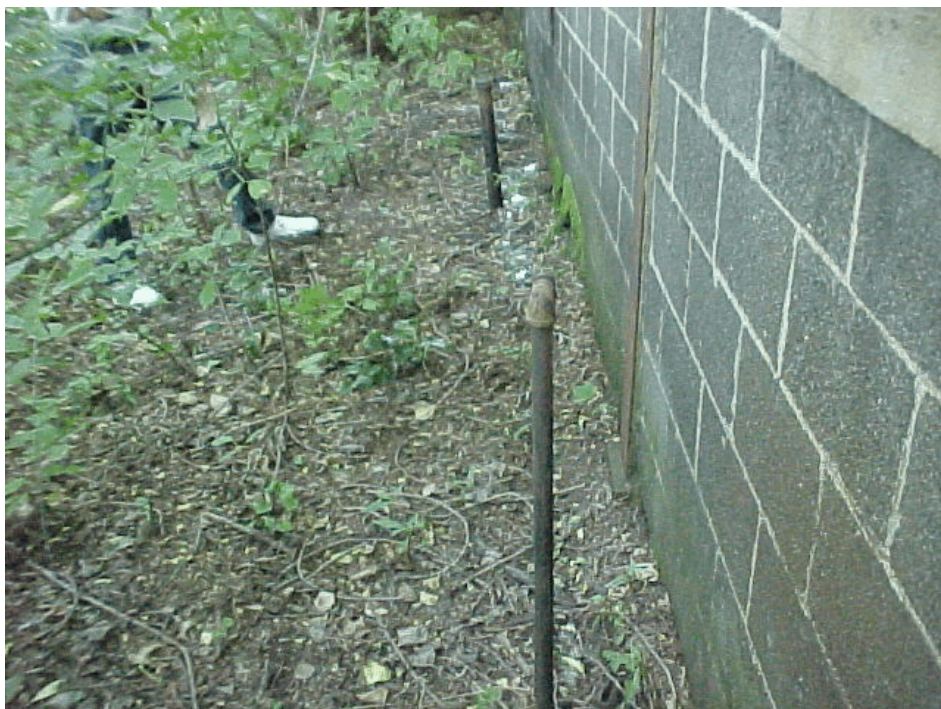
Figure 4-9. Photograph of the fill port and vent for the 4,000 gallon diesel/no. 2 fuel oil USTs behind the Foundry Building. View looking east. Photograph taken by Glenn May on September 18, 2000.
