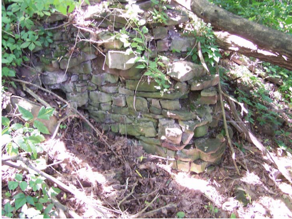
Figure 9-5. Photograph of the historic raceway wall west of the spillway. View looking southwest. Photograph taken by Glenn May on July 14, 2008.
