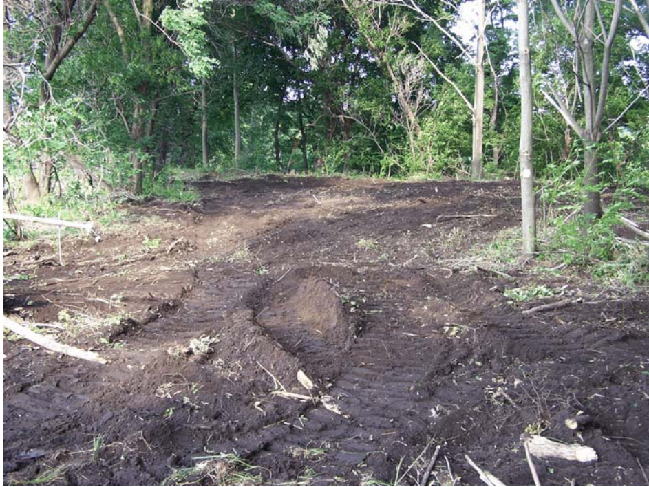
Figure 6-1. Photograph of the foundry sand at the western portion of the Dussault Foundry Site. View looking northwest. Photograph taken by Glenn May on July 28, 2008.
