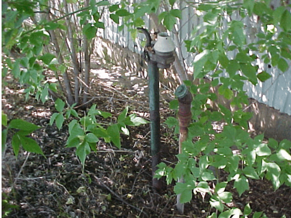
Figure 4-2. Photograph of the fill port and vent for the isopropyl alcohol UST. View looking northwest. Photograph taken by Glenn May on September 18, 2000.
