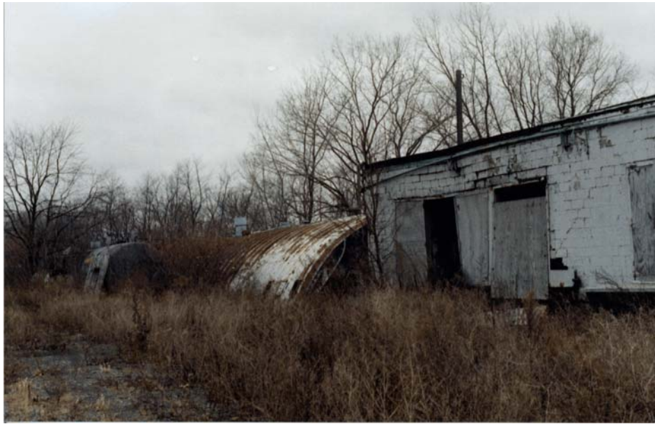
Figure 3-3. Photograph of the dilapidated buildings of the Dussault Foundry Site. The building in the foreground in the Foundry Building, while the metal building in the background is the Quonset Hut. One of the phenolic resin ASTs can also be observed. View looking west. Photograph taken by Ron Voelkel on December 15, 1999.
