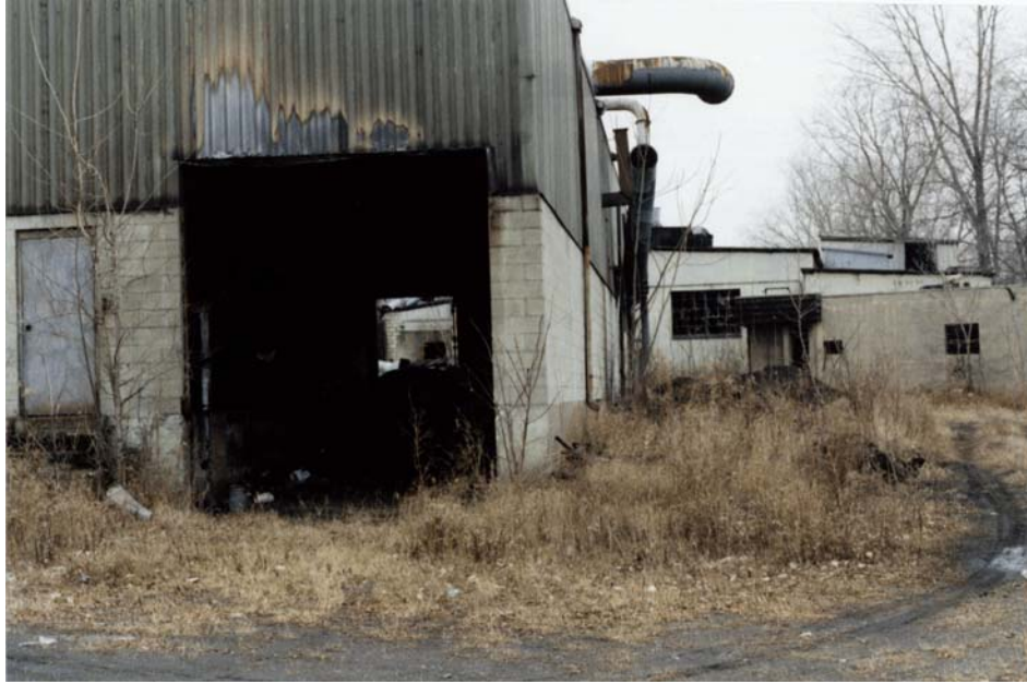
Figure 3-5. Photograph of the dilapidated buildings of the Dussault Foundry Site. The building in the foreground is the Cleaning Building, while the buildings in the background are the Office Building and Area 5. View looking southwest. Photograph taken by Ron Voelkel on December 15, 1999.
