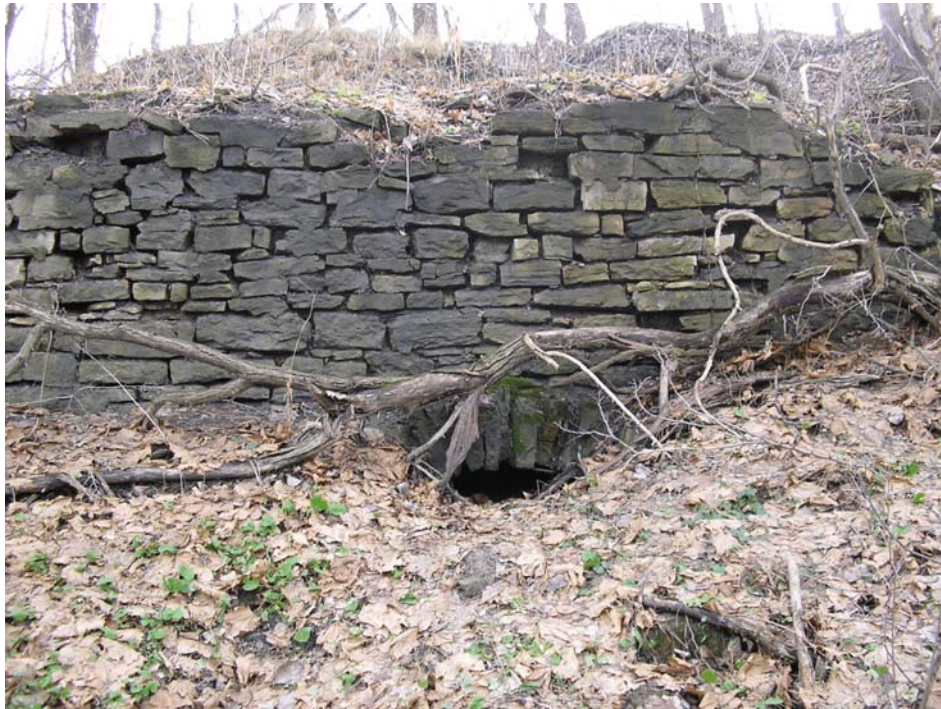
Figure 9-3. Photograph of the historic raceway spillway on the eastern portion of the Dussault property. View looking south. Photograph taken by Glenn May on January 8, 2008.
