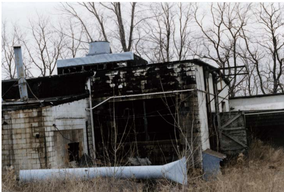
Figure 3-4. Photograph of the dilapidated buildings of the Dussault Foundry Site. The building shown is Area 5. View looking northwest. Photograph taken by Ron Voelkel on December 15, 1999.
