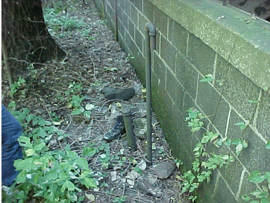
Figure 4-8. Photograph of the fill port and vent for the 1,000 gallon diesel/no. 2 fuel oil UST behind the Foundry Building. View looking east. Photograph taken by Glenn May on September 18, 2000.
