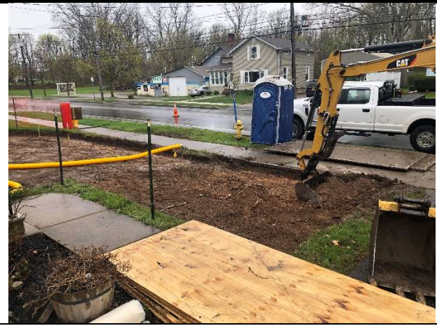
S6: NVES excavating along the west side of the property. View looking southwest.
