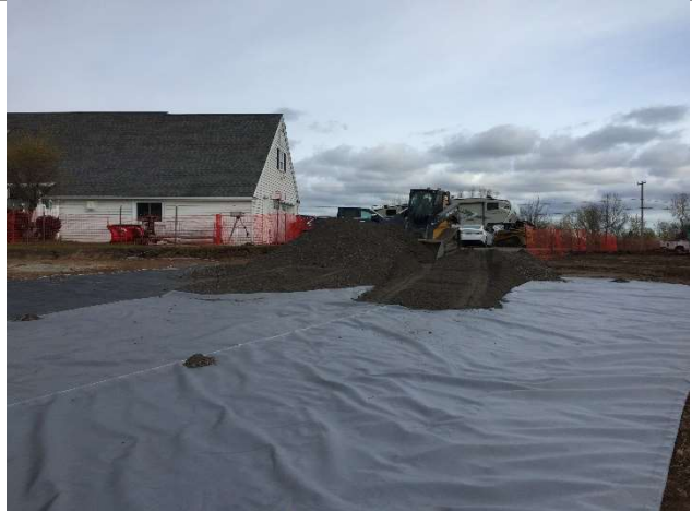
L3: NVES placing stone over geotextile fabric for barn subbase. View looking north.
