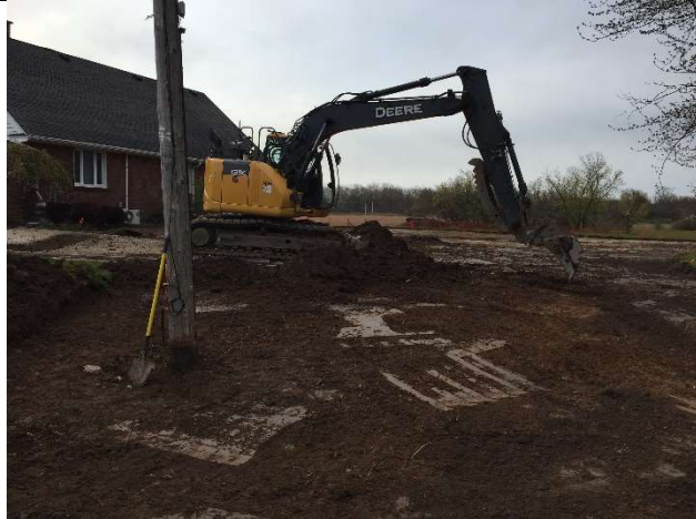
L3: NVES excavating the northwest corner of the property. View looking south.
