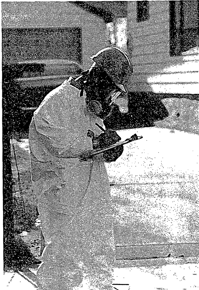
Figure 2. Special protective clothing and equipment is worn by workers nearest the open manholes to protect them from possible exposure to contaminated washwater and sediments.
