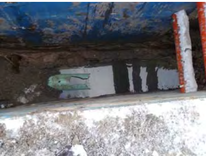
Photo 11: Feb. 03, 2011: Broken PVC pipe and open hole where next section of concrete pipe was removed.
