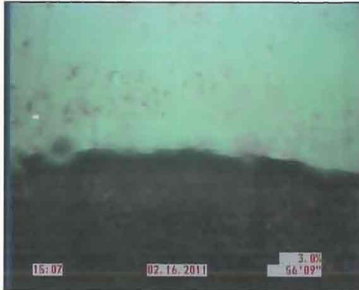
Photo: 4_1_2_17022011_140929_A.JPG, VCR No.: X 56.75FT, Material Change, Concrete pipe (non-reinforced) / PVC (SDR35) to Concrete
