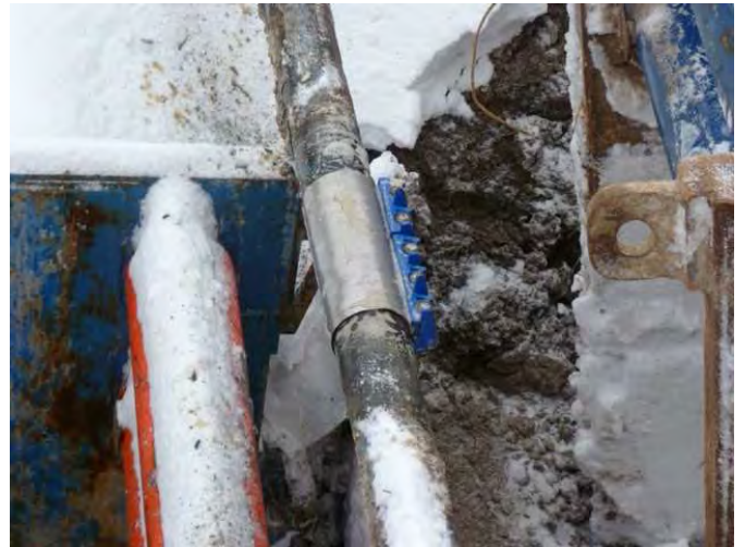
Photo 4: Feb. 02, 2011: Gas line was discovered to be leaking. National Fuel Gas repaired with a sleeve.
