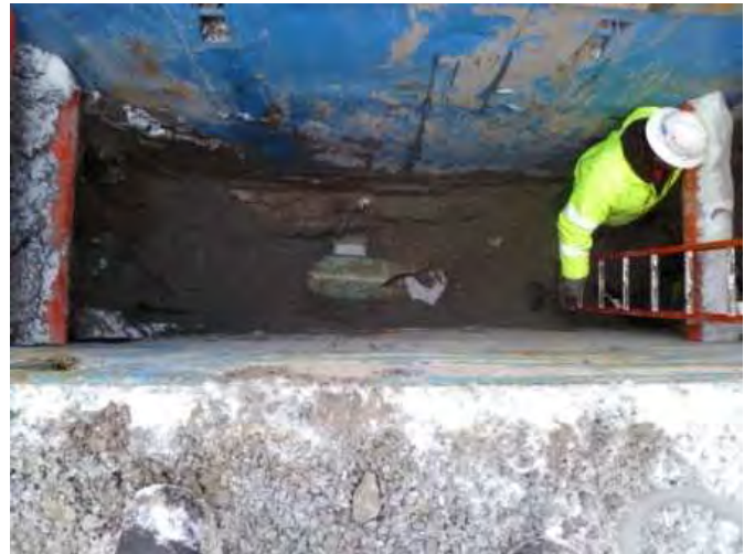
Photo 10: Feb. 03, 2011: Broken PVC sanitary sewer pipe; was supposed to be concrete pipe.
