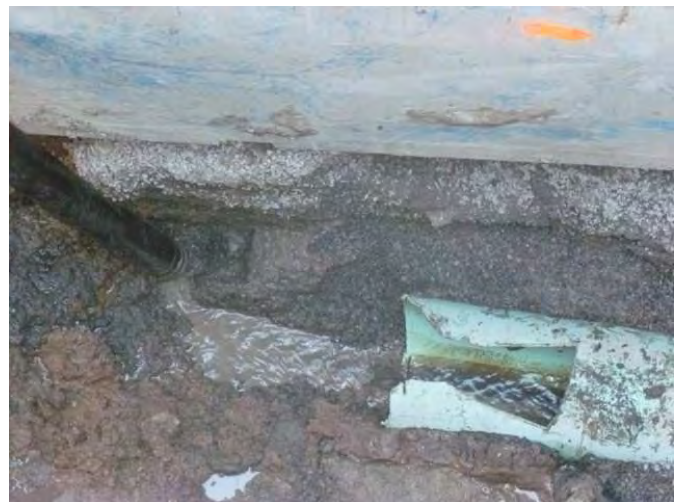
Photo 12: Feb. 04, 2011: Vacuuming water from excavation; water coming from the sanitary sewer pipe.
