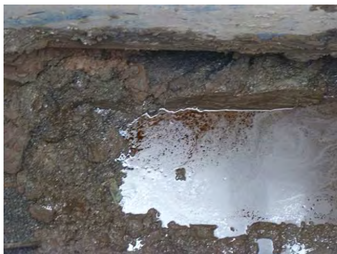
Photo 34: Feb. 10, 2011: Stained gravel and NAPL-like material prior to removal to extent possible. Distance from manhole at 96 th Street is approximately 38 ft to the east.
