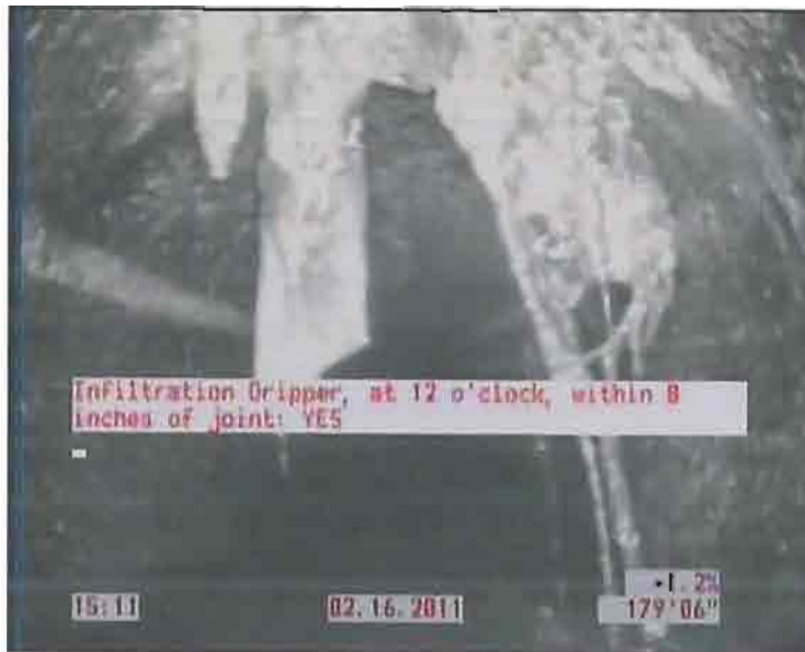
Photo: 4_1_3_17022011_141402_A.JPG, VCR No.: X 179.5FT, Infiltration Dropper, at 12 o'clock, within 8 inches of joint: YES / Infiltration
