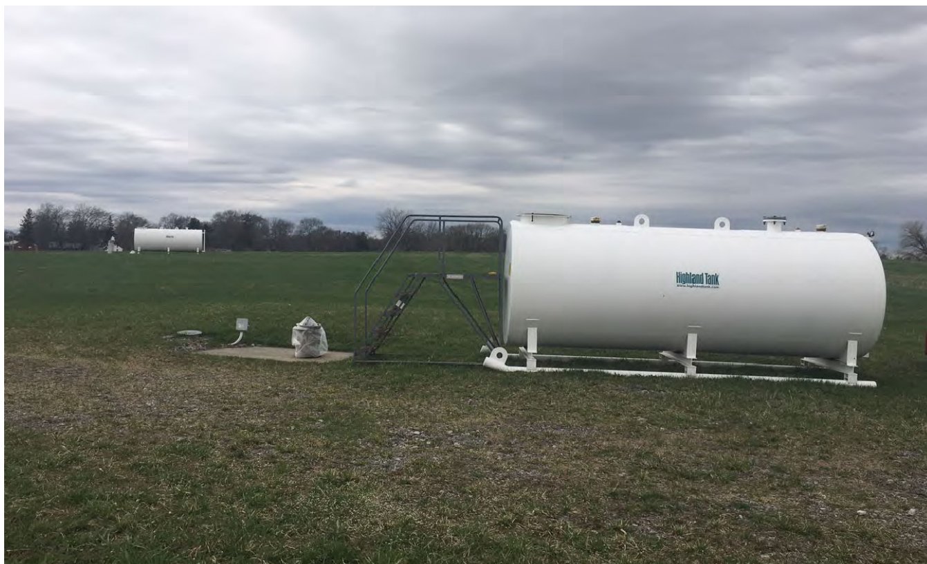
Figure 18: 2,500 gallon skid tanks.
