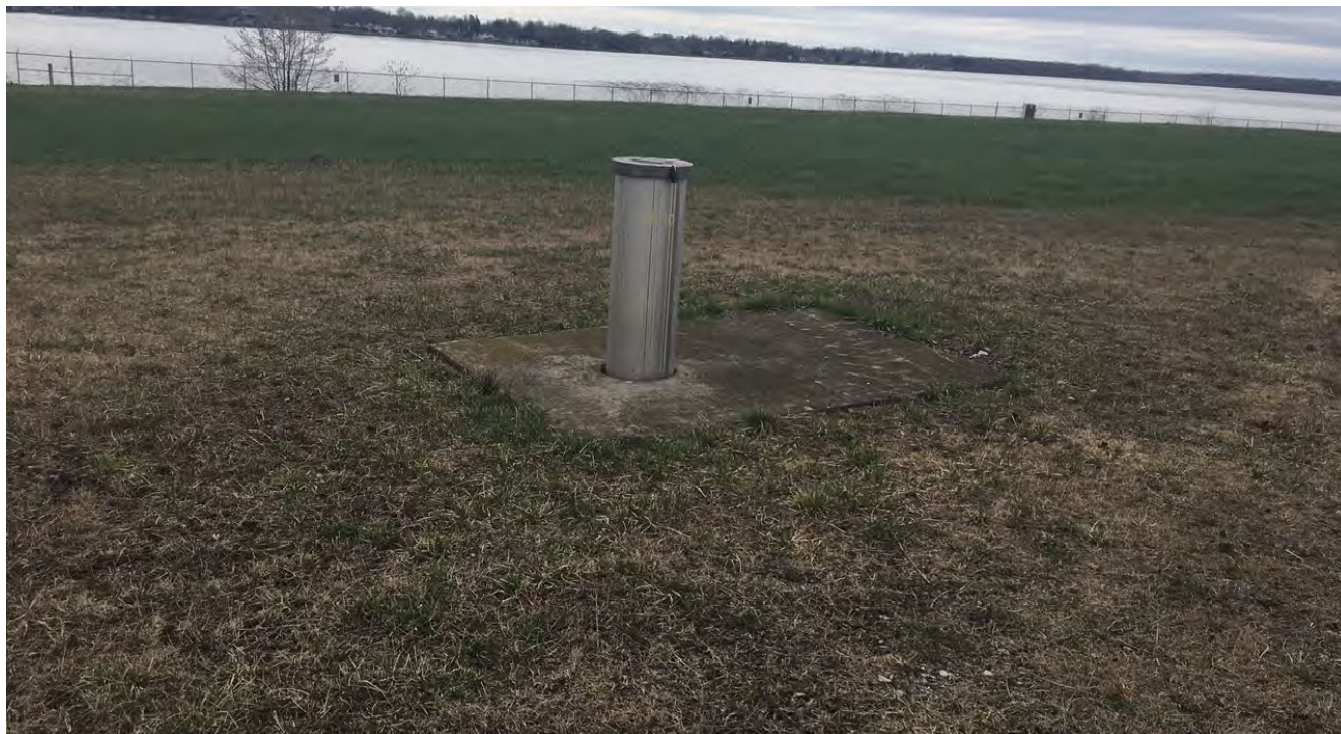
Figure 20: Closeup of a NAPL recovery well.
