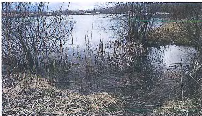
Inundated Overflow Weir
