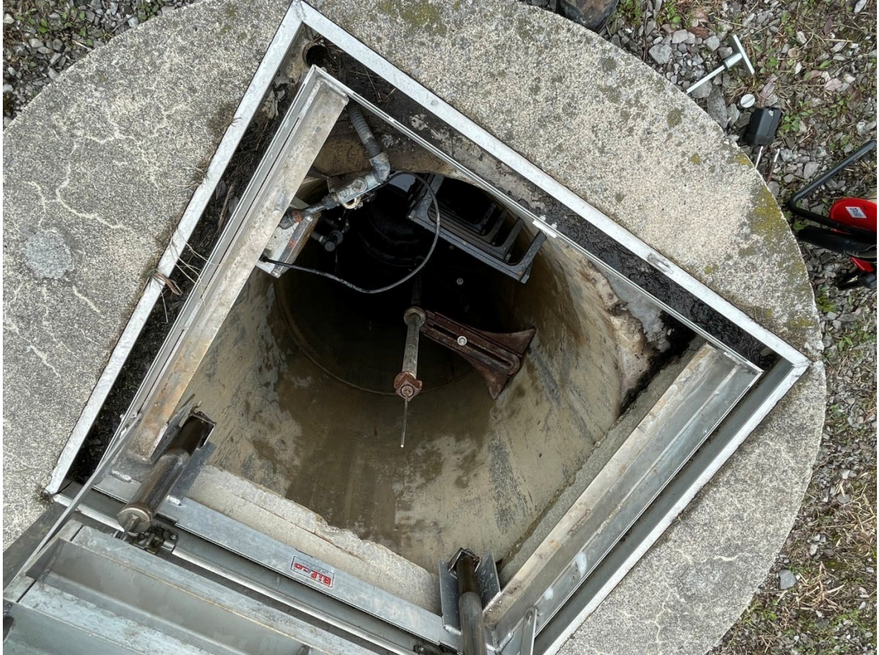
Groundwater collection system sump vault.
