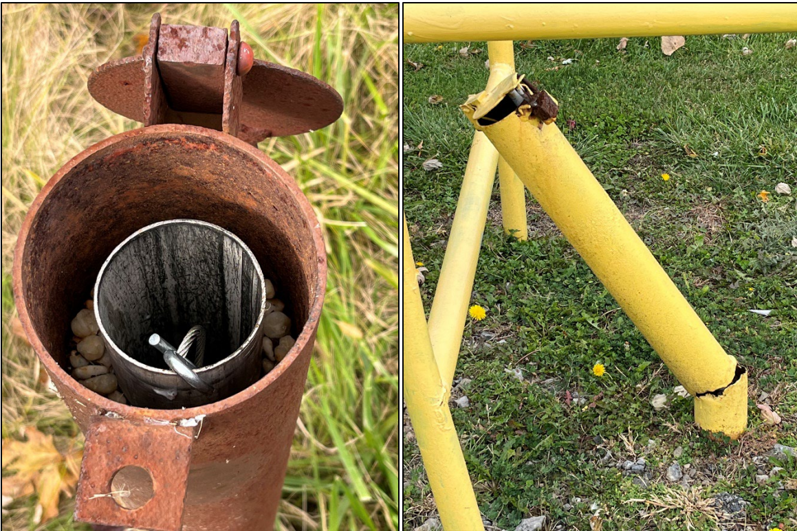
On 10-24-2024, 87-19(1) wellhead showing cable used to hang new HydraSleeve sampler in well (left). During site reconnaissance, damage was observed to well 86-23A on Walmore Road near the southernmost parking lot entry (right).
