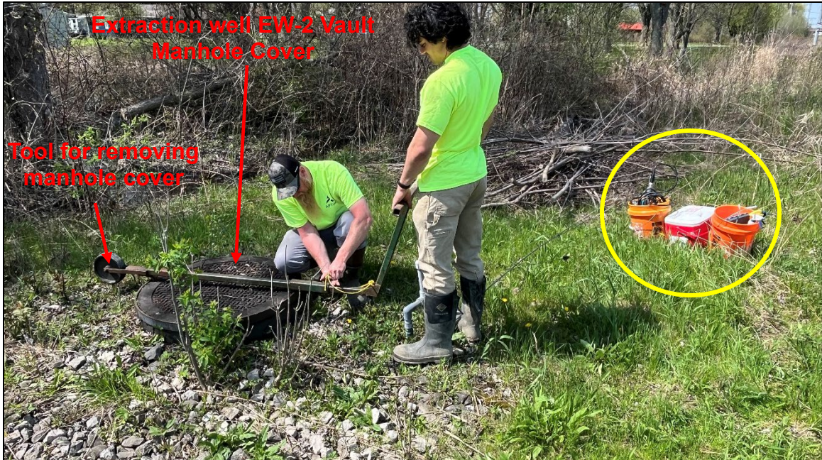
APTIM personnel removing the manhole cover on extraction well EW-2 using specialized tool; sampling equipment in right of photo (yellow circle).
