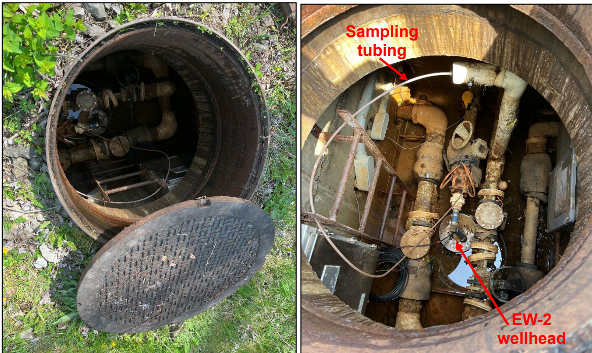
Views of inside of extraction well EW-2 vault. Wellhead and sampling port tubing shown in right photo.
