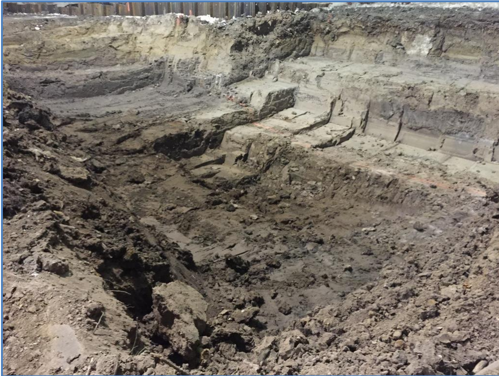
Figure I-22. Photo showing the upper sand deposit (yellow-brown) and the underlying silty clay deposit (brown and reddish-brown) in the IRM excavation area. Photo taken by Kevin Glaser on February 27, 2015.
