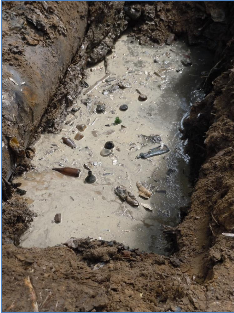
Figure I-4. Photo showing landfill waste in a test pit completed on National Fuel Gas property west of the main Niagara Sanitation landfill. Photo taken by Steven Moeller on July 20, 2020.
