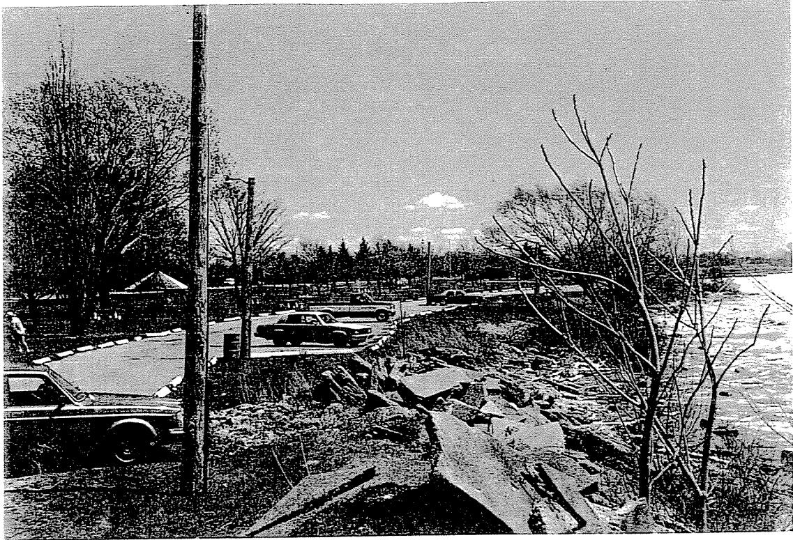
Photo 13 - Western section of park shoreline facing southeast from a point 40 ft west of the west park access road and 30 ft from shore.
