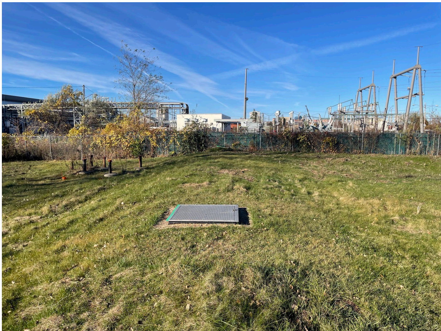
Pumping well cover.
