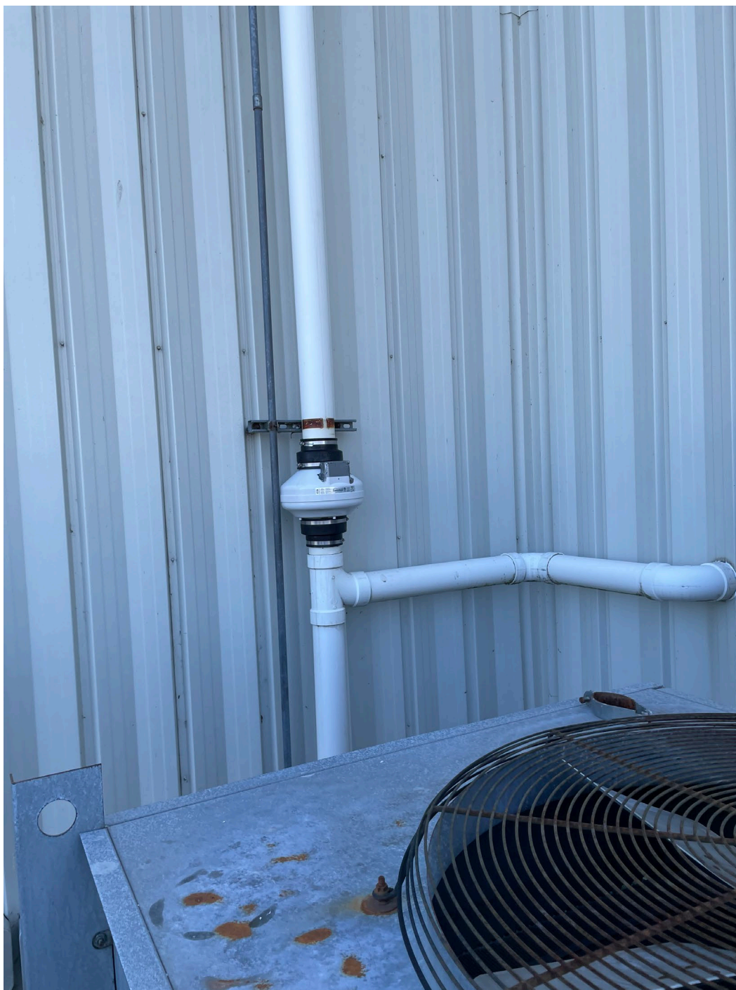
SSDS line outside on NE corner of building.
