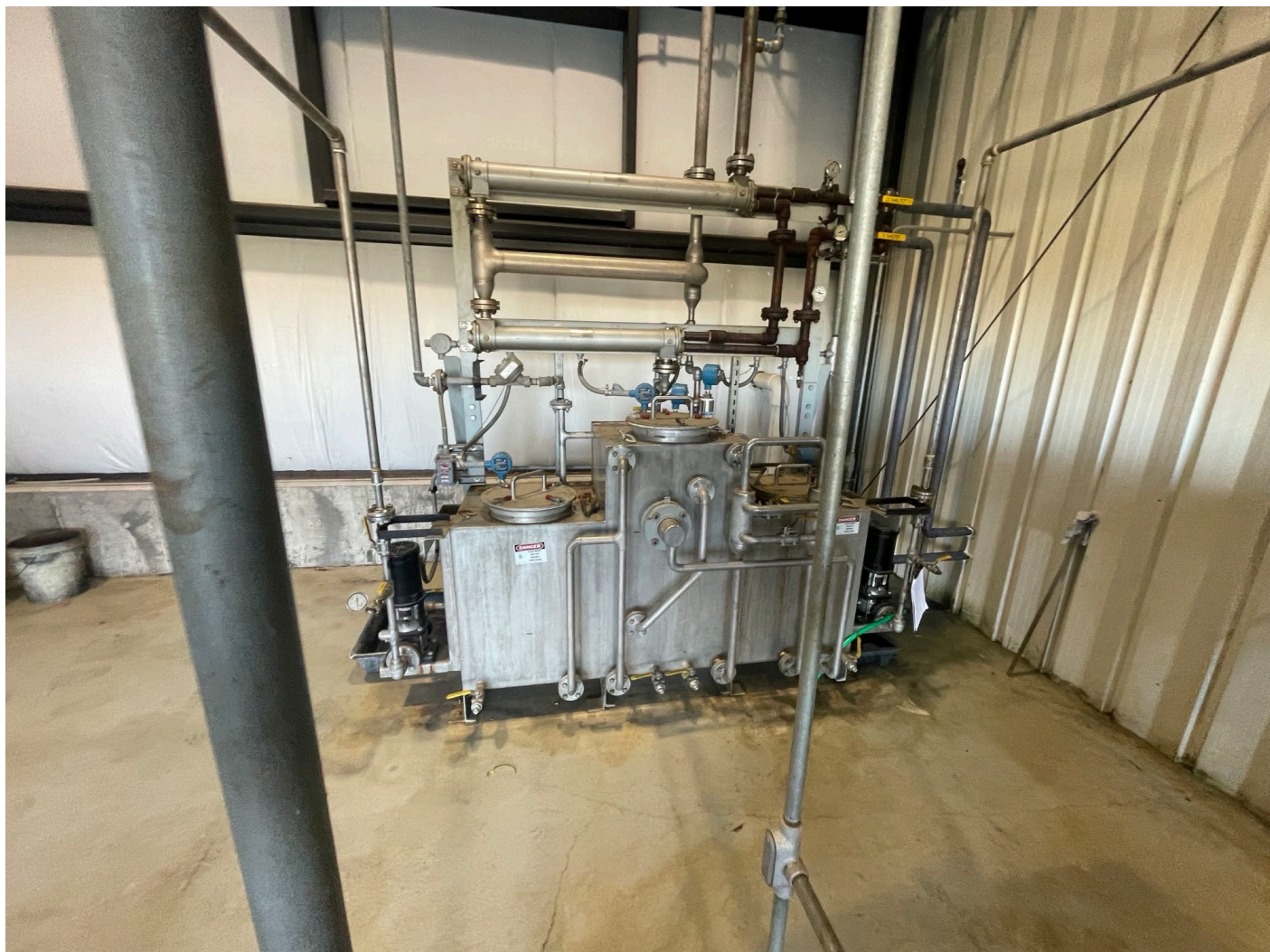
Oil-water separator system.
