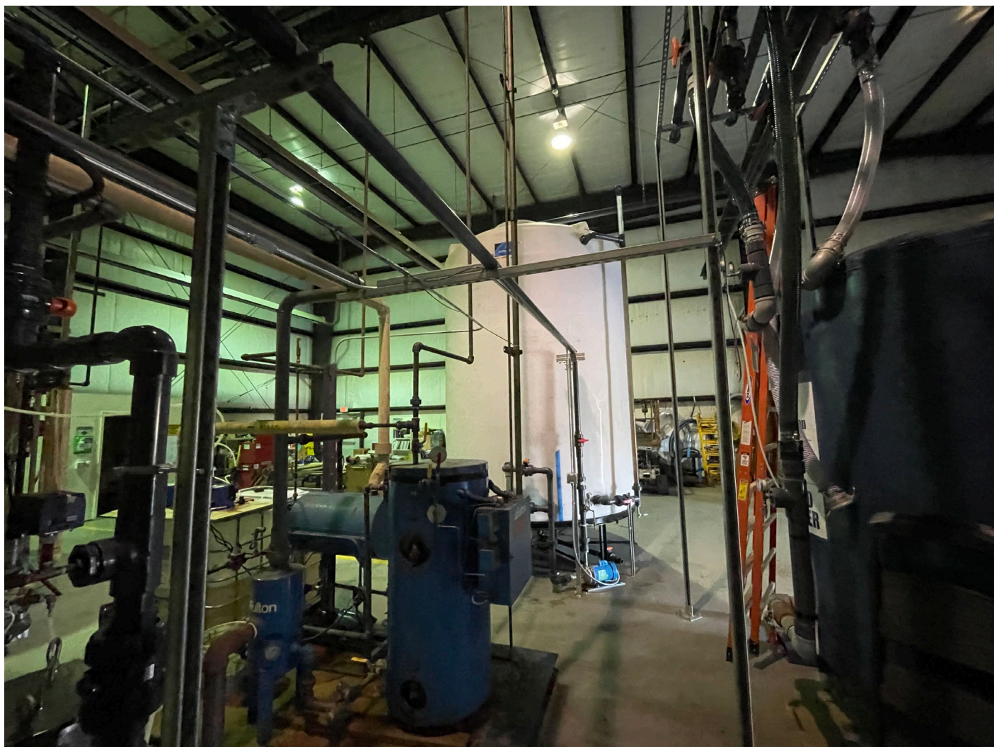
Backwash tank (white).
