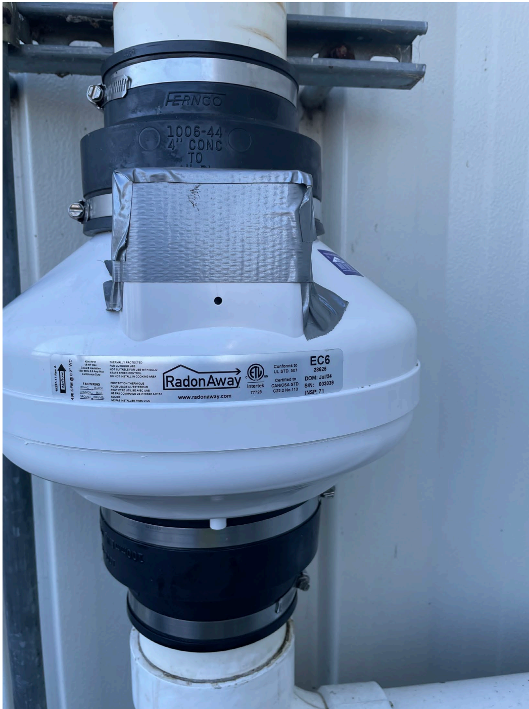
Electric fan recently installed per TRC (was a passive vent type fan previously).
