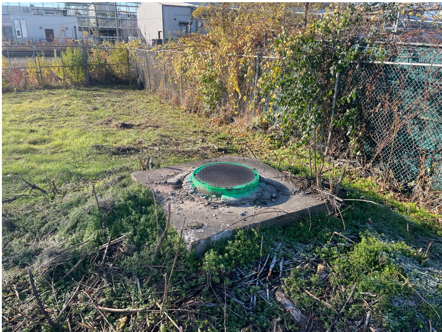
Pumping well cover.
