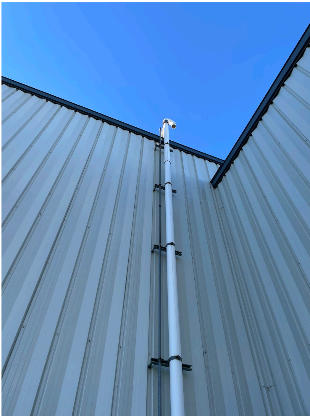
SSDS exhaust to roof with downward facing end.
