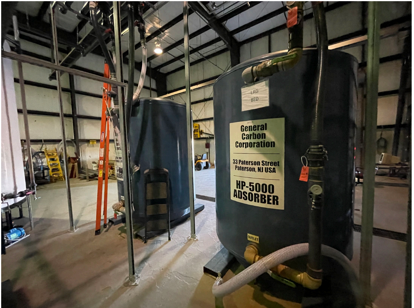
Carbon beds added during modifications to stricter Niagara Falls Water Board pretreatment thresholds.
