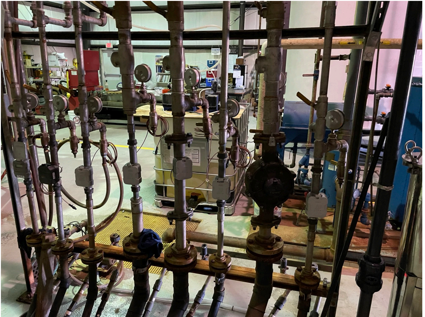
Pumping well intake lines.
