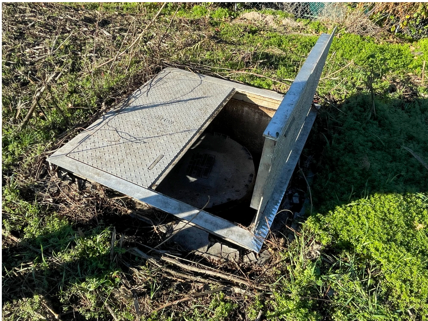
Pumping well cover for manhole access.
