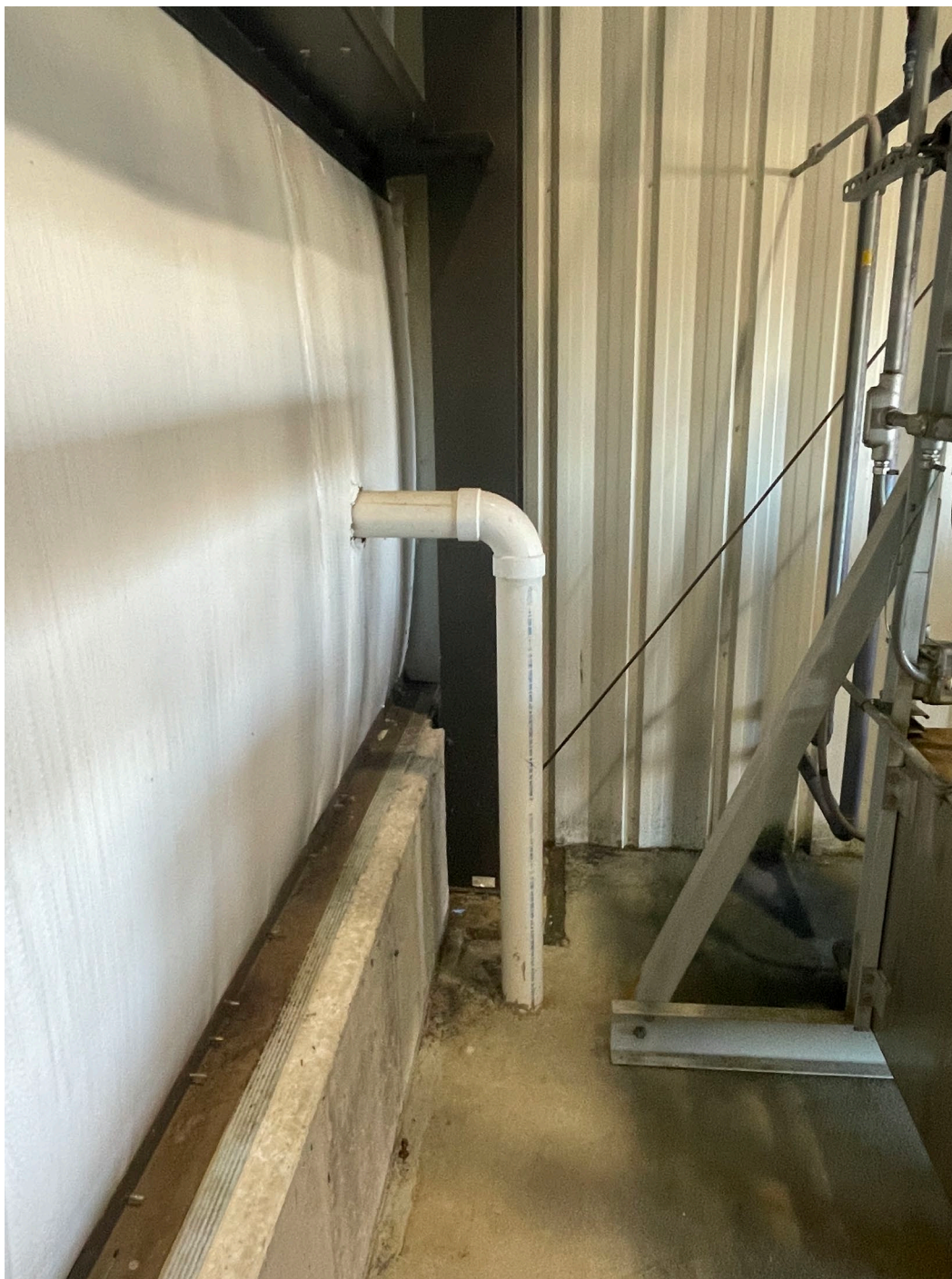
SSDS line entering sub-slab.
