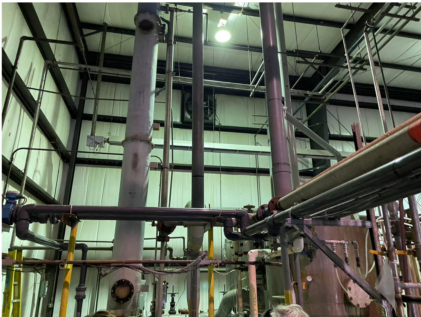
Air stripper recirculating/exhaust lines.
