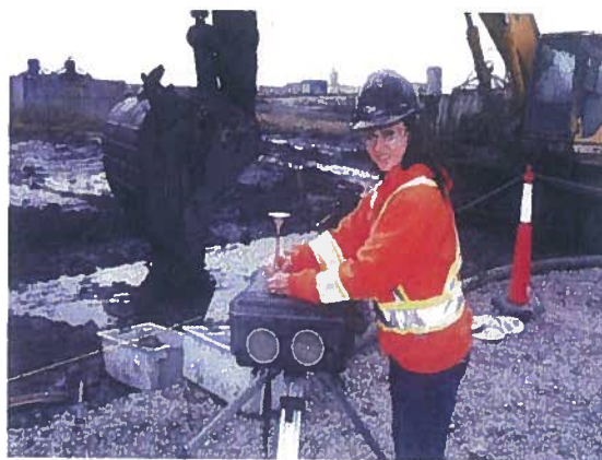
Engineer checks air evaluation monitor
