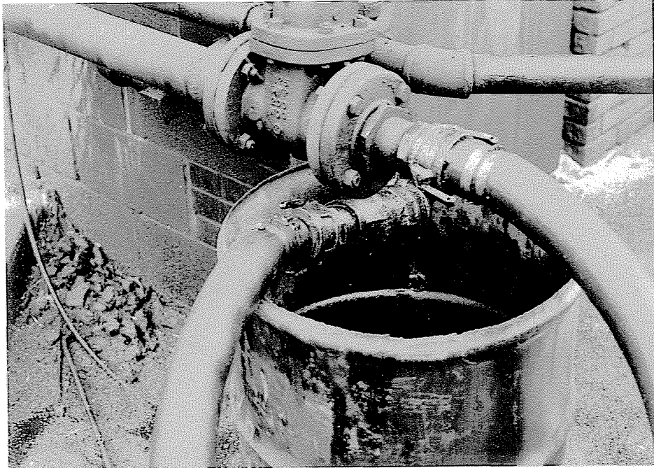
UNLOADING LINE HOSE DRAININGS
