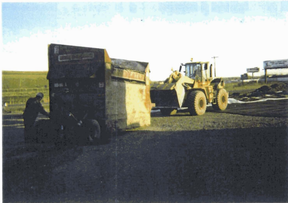
READ SCREEN ALL USED FOR SEGREGATING MATERIAL
