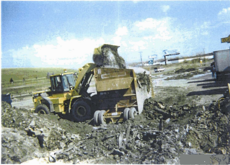
SCREEN IN OPERATION
