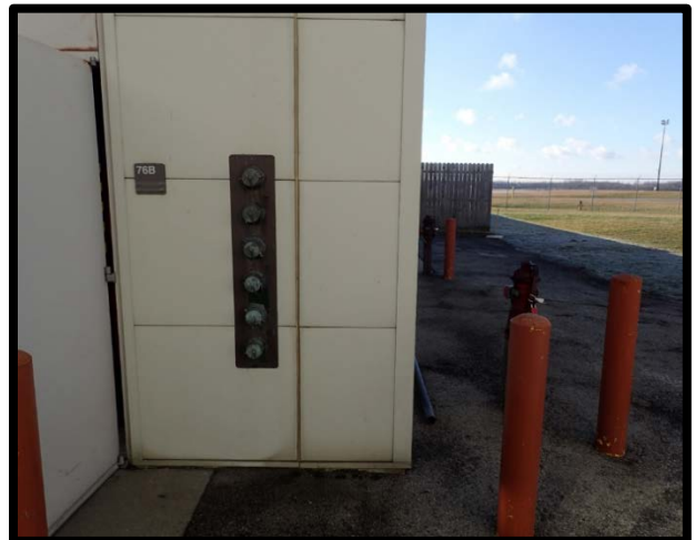
Photo 18 Building 907 external manifold.
