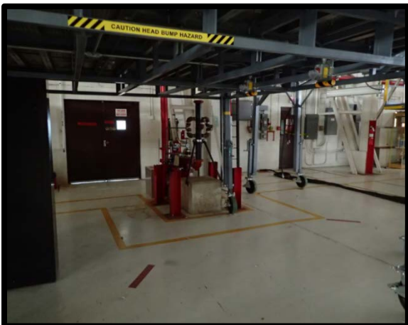
Photo 47 Building 850 AFFF dispensing system.
