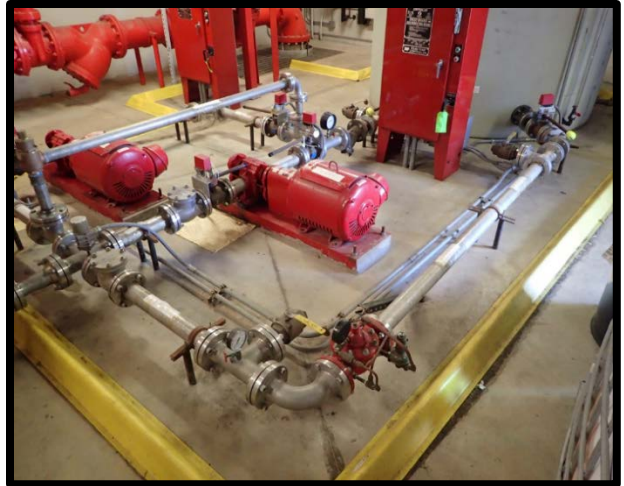
Photo 50 AFFF feed system in Building 707.
