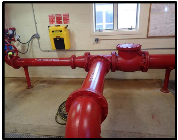
Photo 34 Building 850 AFFF dispersion system.
