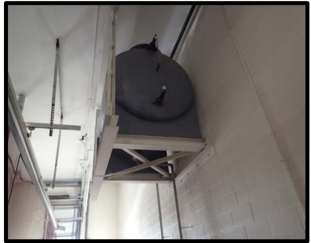
Photo 10 1,000-gallon AFFF storage tank.
