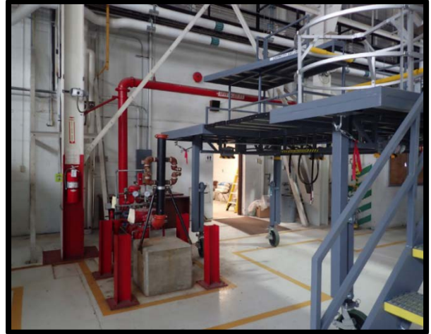
Photo 44 Building 850 AFFF dispensing system.
