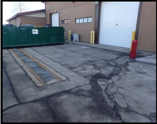
Photo 79 Building 700 (old fire station), drains not on the flight side
