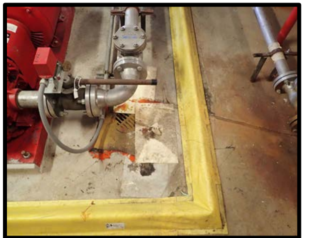
Photo 54 - Leaking flanges in Building 707.
