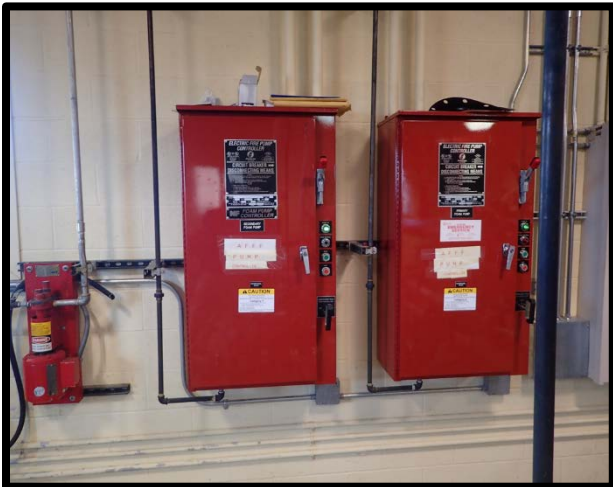
Photo 39 - Building 850 fire control system.
