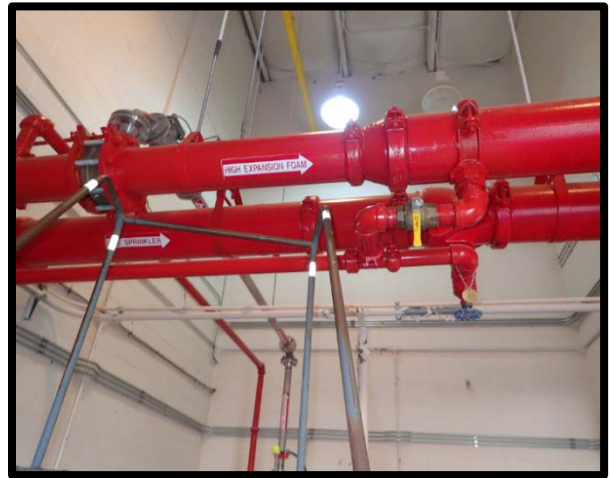
Photo 28 Building 917 Hi Ex dispersion pipes.
