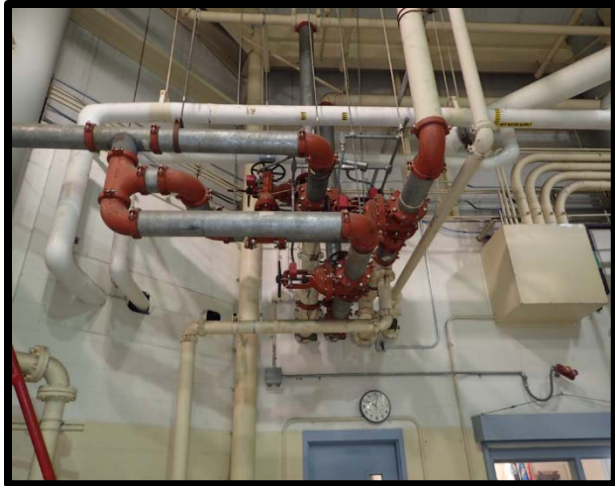
Photo 19 AFFF dispersion manifold.
