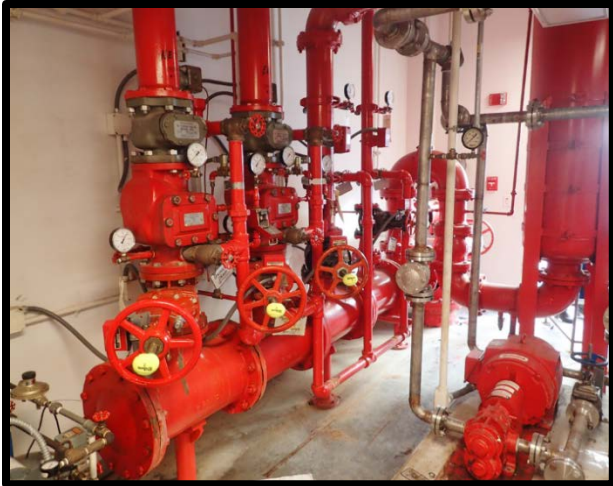
Photo 13 Building 907 AFFF dispensing system.
