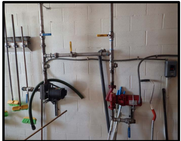
Photo 12 AFFF storage tank dispenser.
