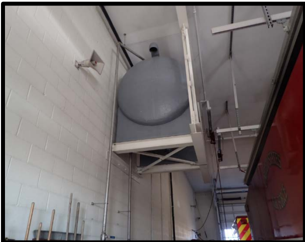
Photo 11 AFFF storage tank at Building 821.
