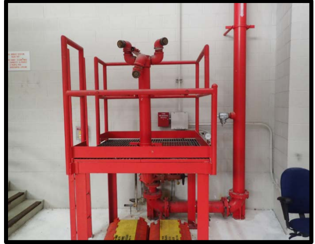
Photo 56 Building 707 AFFF dispersion system.
