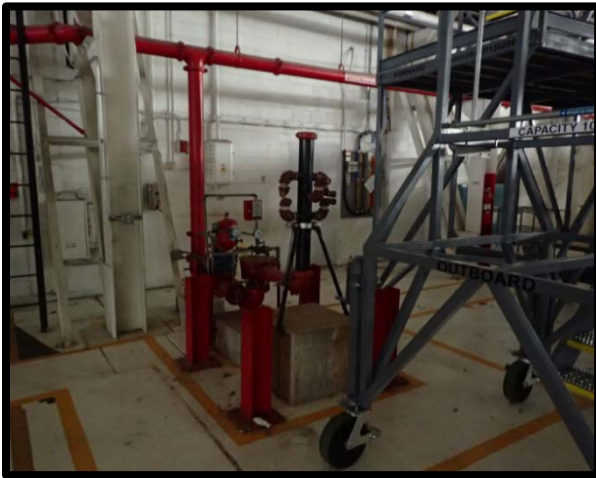
Photo 45 Building 850 AFFF dispensing system.
