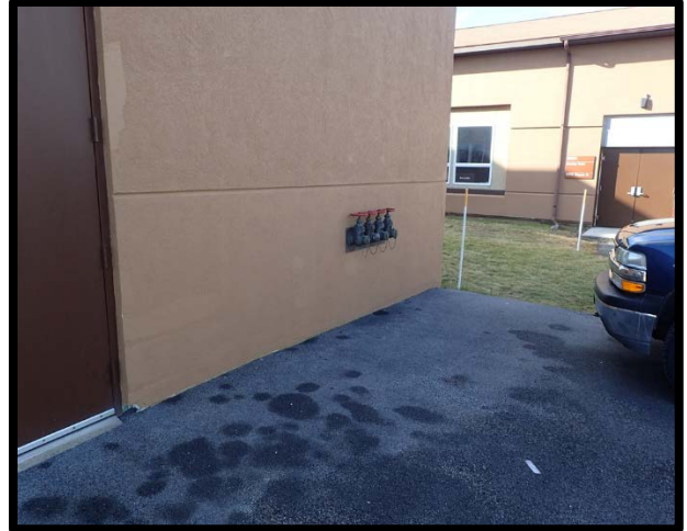
Photo 38 Building 850 external manifold.
