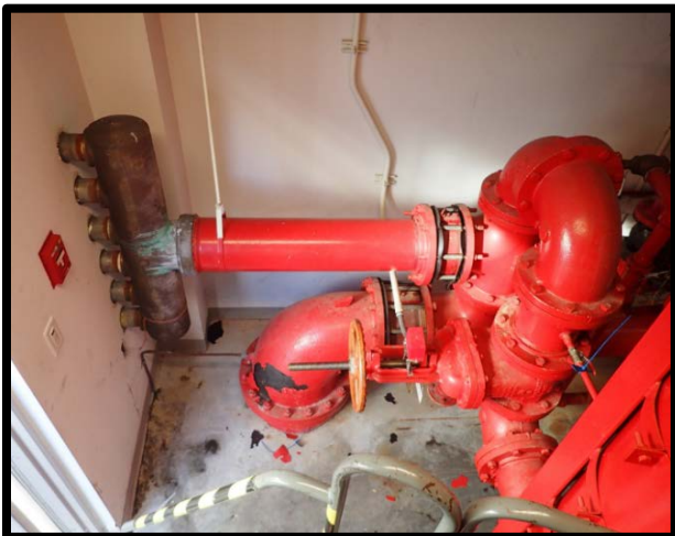
Photo 17 Building 907 external manifold.
