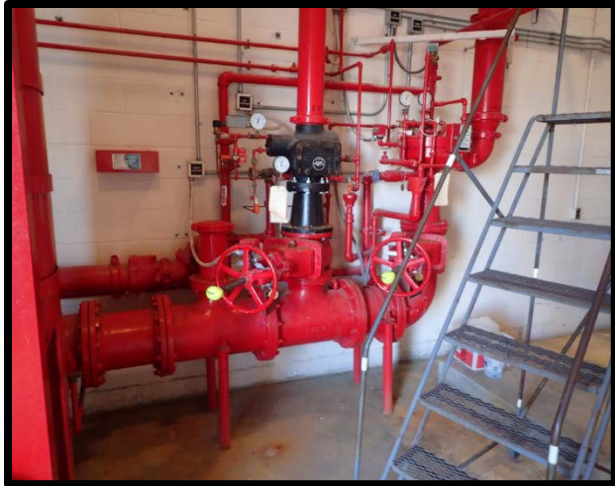
Photo 31 Building 917 Hi Ex system.
