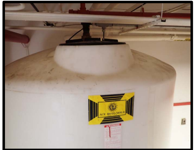
Photo 16 Building 907 top of AFFF tank.
