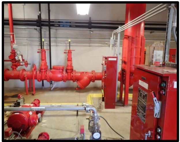
Photo 52 Building 707 AFFF water main supply.
