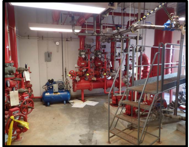
Photo 14 Building 907 AFFF dispensing system.
