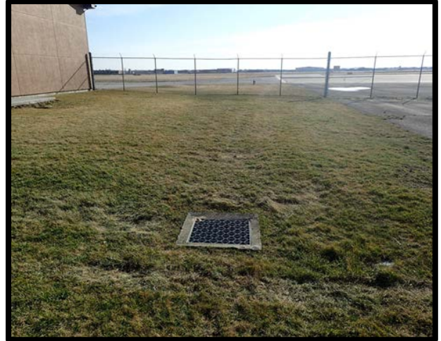
Photo 80 East side of Building 700 (note the drains that connect to those on the runway apron).
