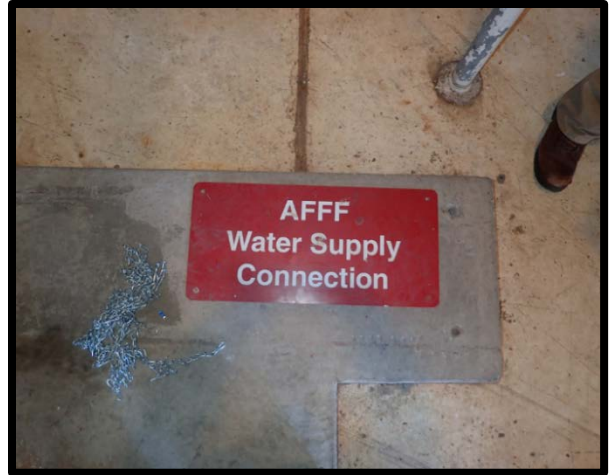
Photo 26 AFFF sign found on floor of Building 917.
