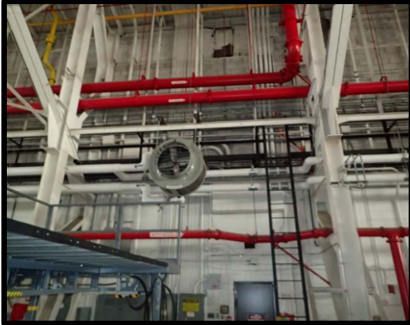
Photo 43 Building 850 fire suppression system.
