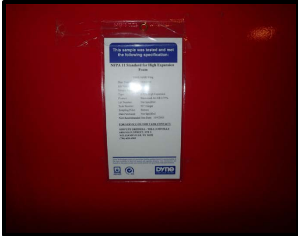
Photo 25 - Building 917 Hi Ex tank label.
