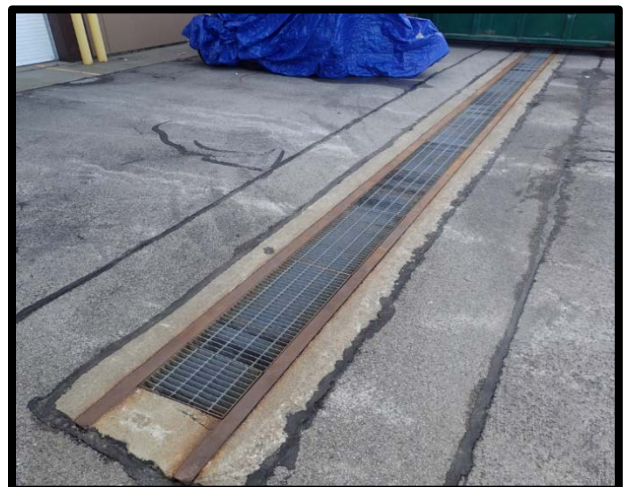
Photo 78 Building 700, drains not on the flight side.
