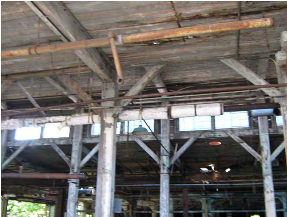
Photograph 2 – PACM covered pipe in the north building.
