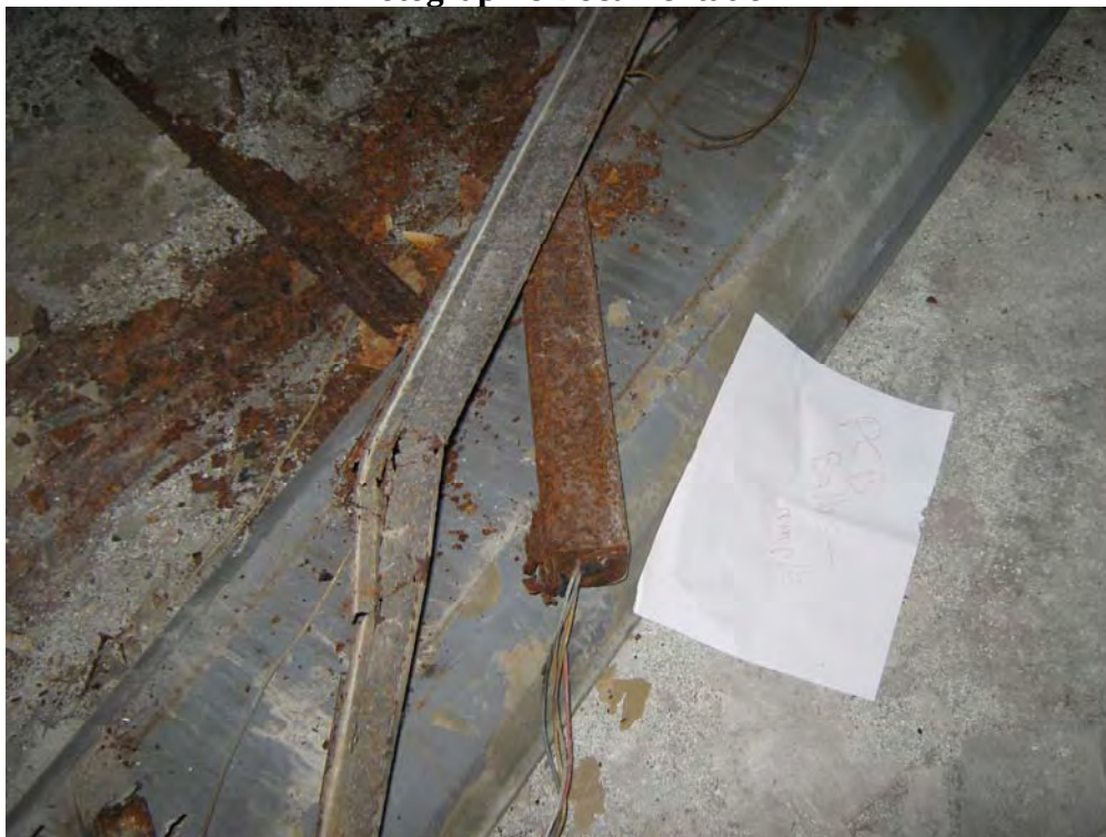
Photograph 9 – One of several light ballasts observed in the building. Two light ballasts were collected and submitted for PCBs analysis.
