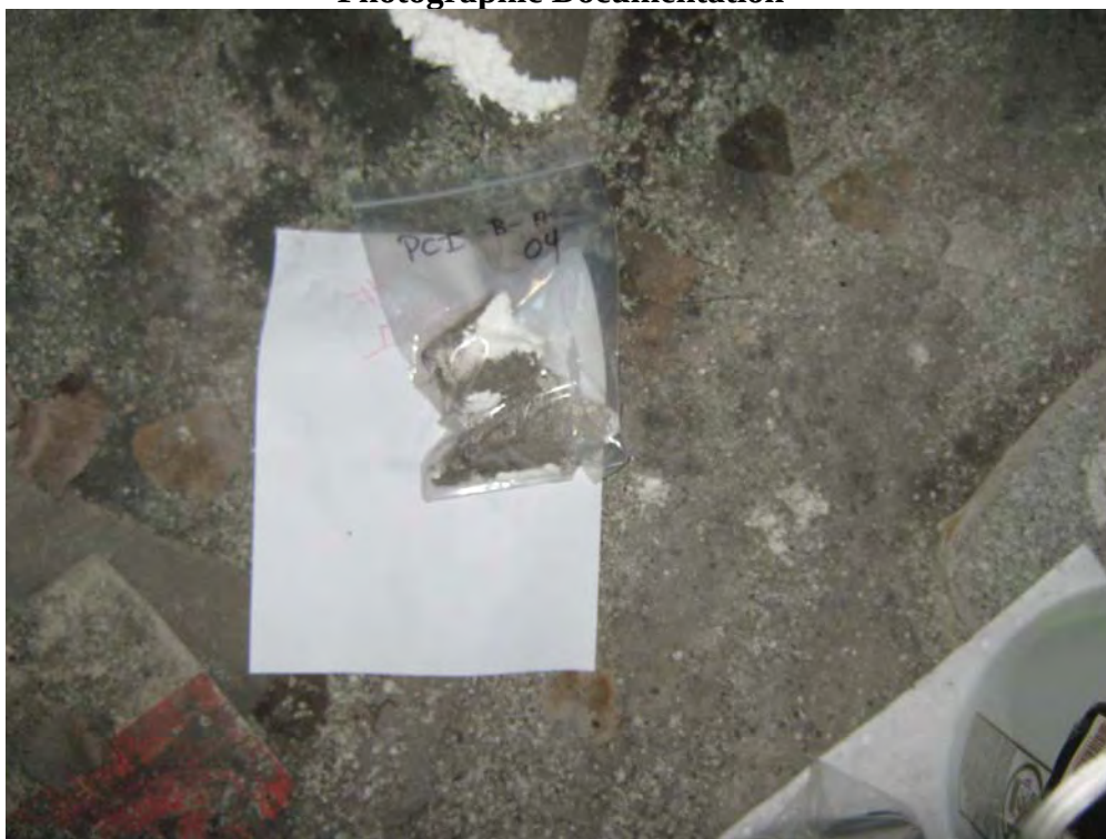
Photograph 5 – Sample PC1-B-AS-04 collected from PACM on the floor and submitted for asbestos analysis.
