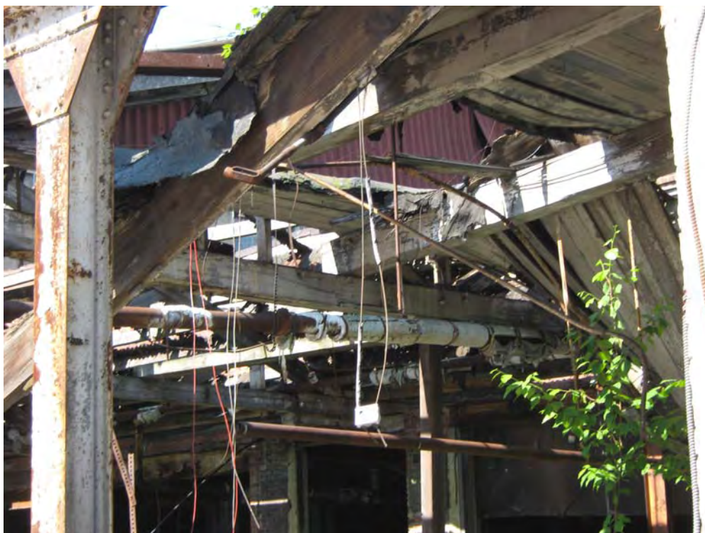
Photograph 10 – Eastern end of the building where the roof had collapsed. The picture was taken from outside the building. Deteriorated PACM is seen and is exposed to the outside air.
