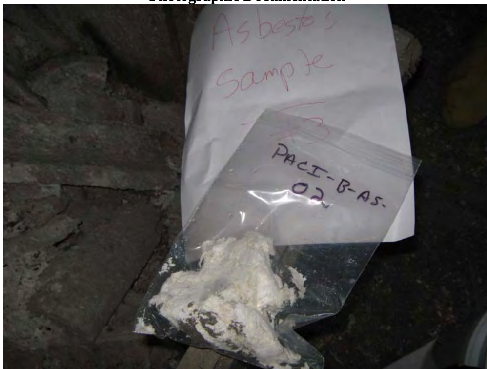
Photograph 3 – Sample PC1-B-AS-02 collected from PACM on the floor and submitted for asbestos analysis.
