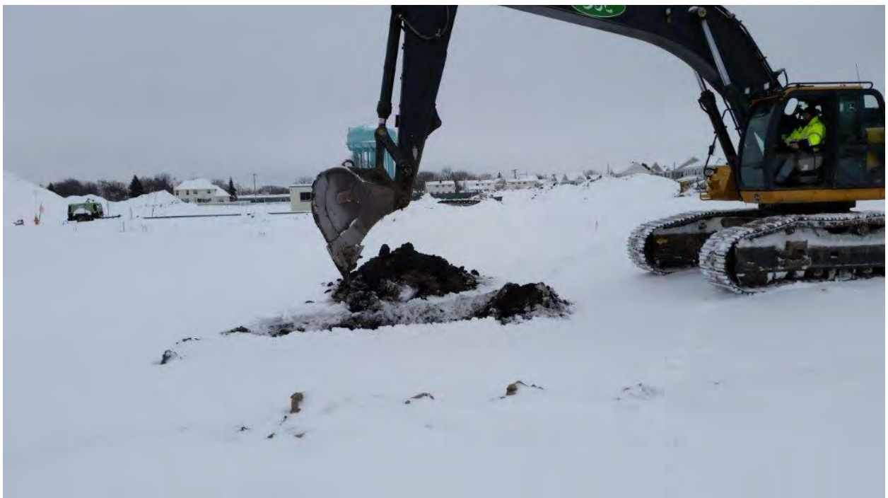
Re-excavation at test pit LNAPL-1 on February 10, 2015. Photo and description provided by AMEC.
