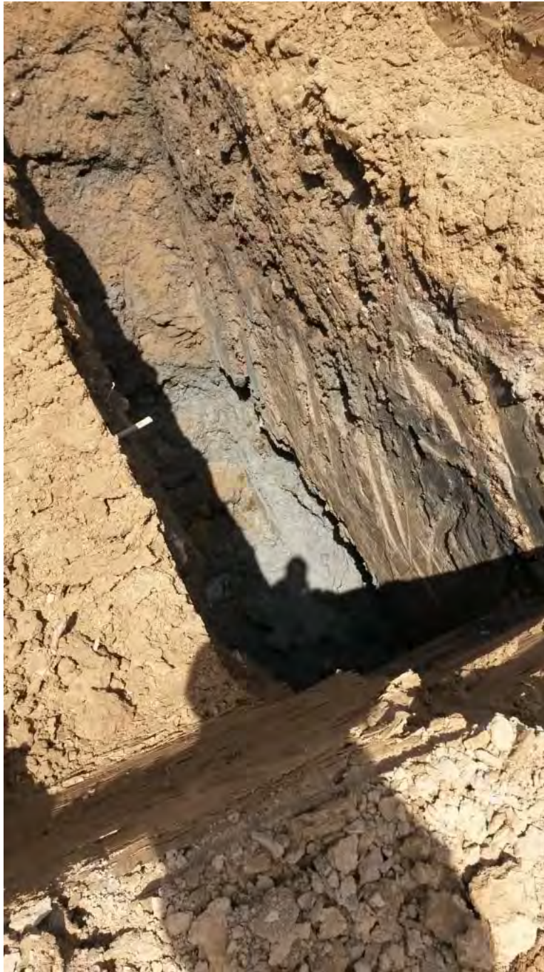
View of test pit LNAPL-21 during advancement on April 24, 2015. No NAPL impacts were observed.
