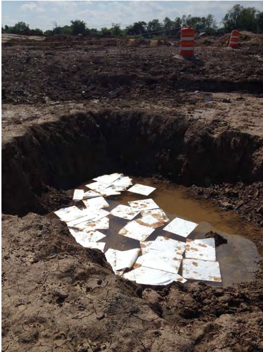
View of hydrophobic sorbent pads on surface of test pit used for the collection of NAPL in May 2015.
