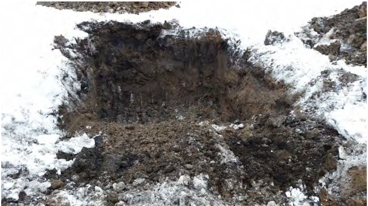
Test pit LNAPL-1 widened to three bucket-widths (as NAPL impact not as prominent as was observed on February 3, 2015). Photo and description provided by AMEC.
