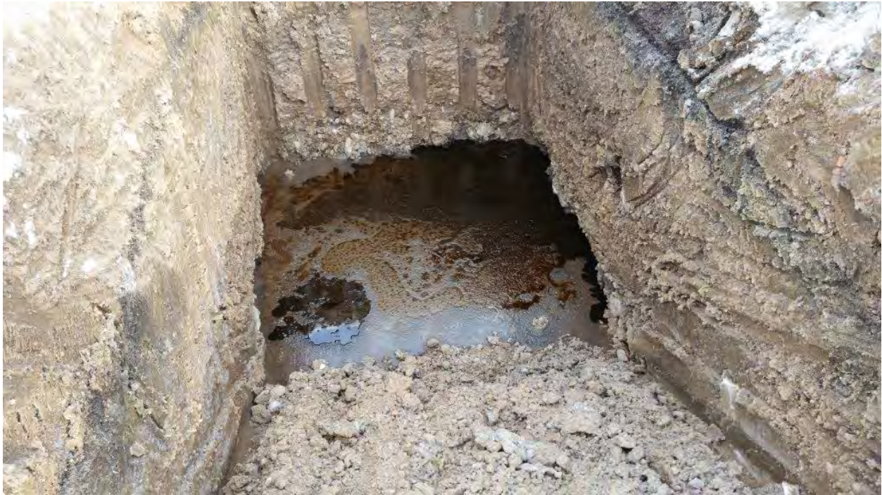
Accumulation of NAPL in test pit LNAPL-2 one day after excavation. Photo and description provided by AMEC.
