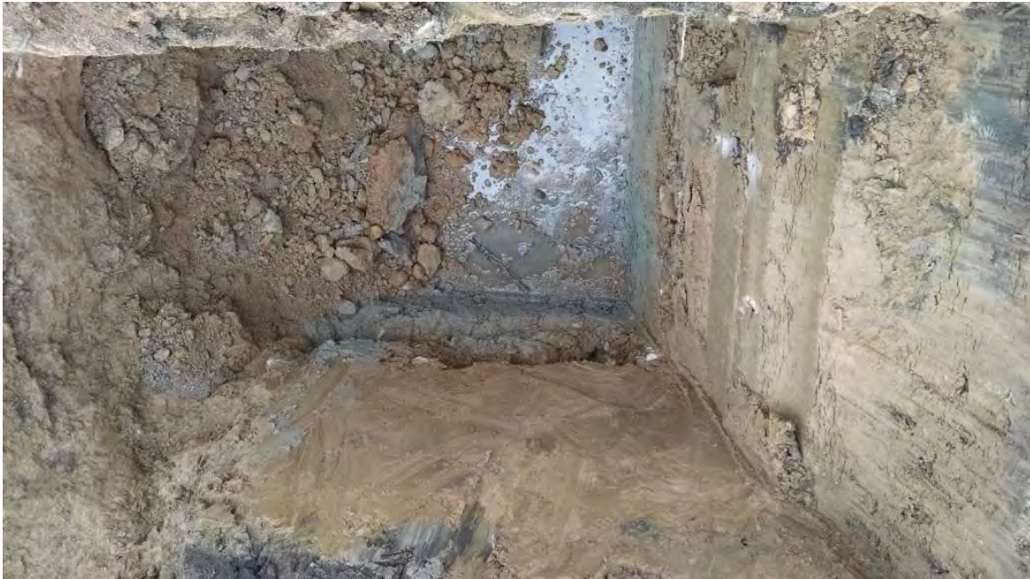
View of test pit LNAPL-14 upon completion on April 23, 2015, showing sheen on water at bottom of test pit.
