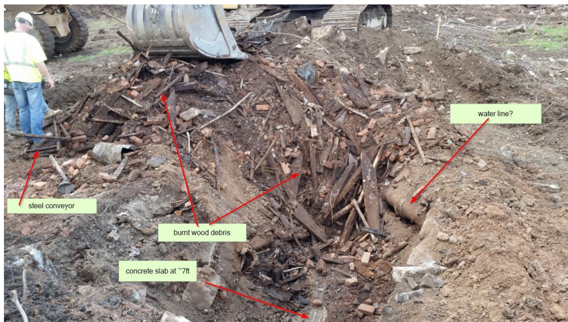
Photo 2: Burnt building debris in Western Commercial Area
