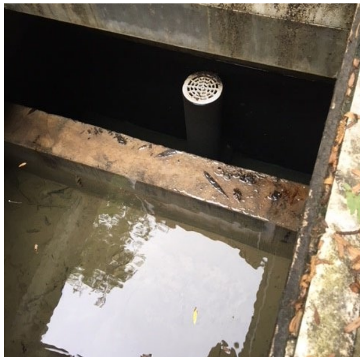
Photo 2: Interior of filter vault – overflow in discharge chamber (November 25, 2019).
