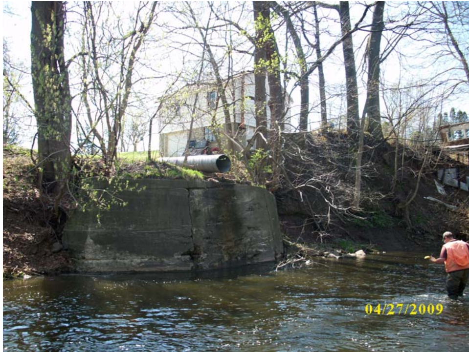
Photo: P125 Direction of view: SE Description: Drainage pipe along RDB, old abutment (OUT-023).
