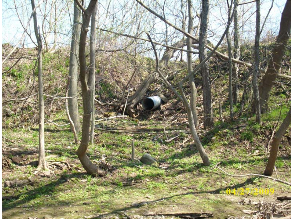
Photo: P72 Direction of view: NE Description: Drainage pipe along RDB (OUT-024).
