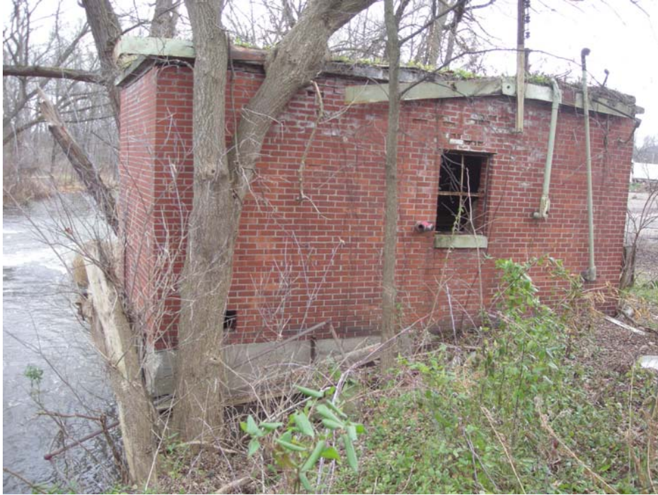
Photo: P56A Direction of view: N Description: Pump house on RDB.
