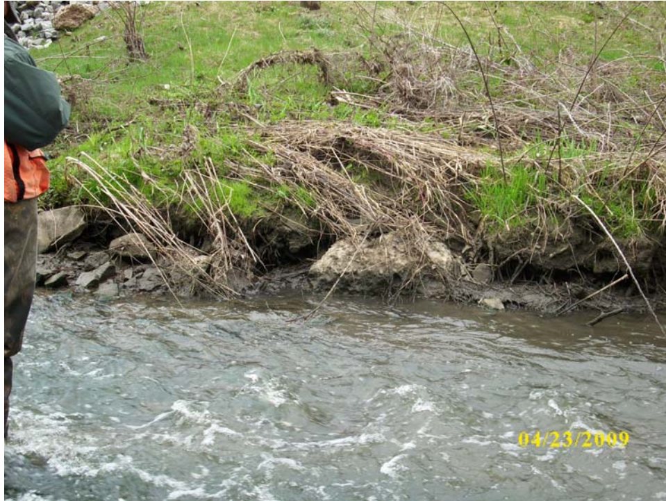
Photo: P22 Direction of view: SW Description: Seepage along LDB (DRN-021).
