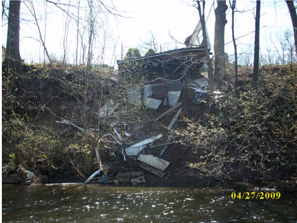
Photo: P69 Direction of view: SW Description: Dilapidated structure along RDB.
