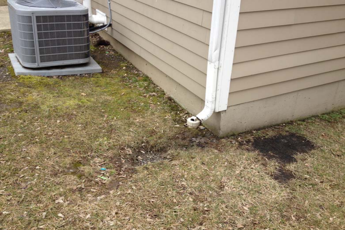
Minor erosion around drain pipe
