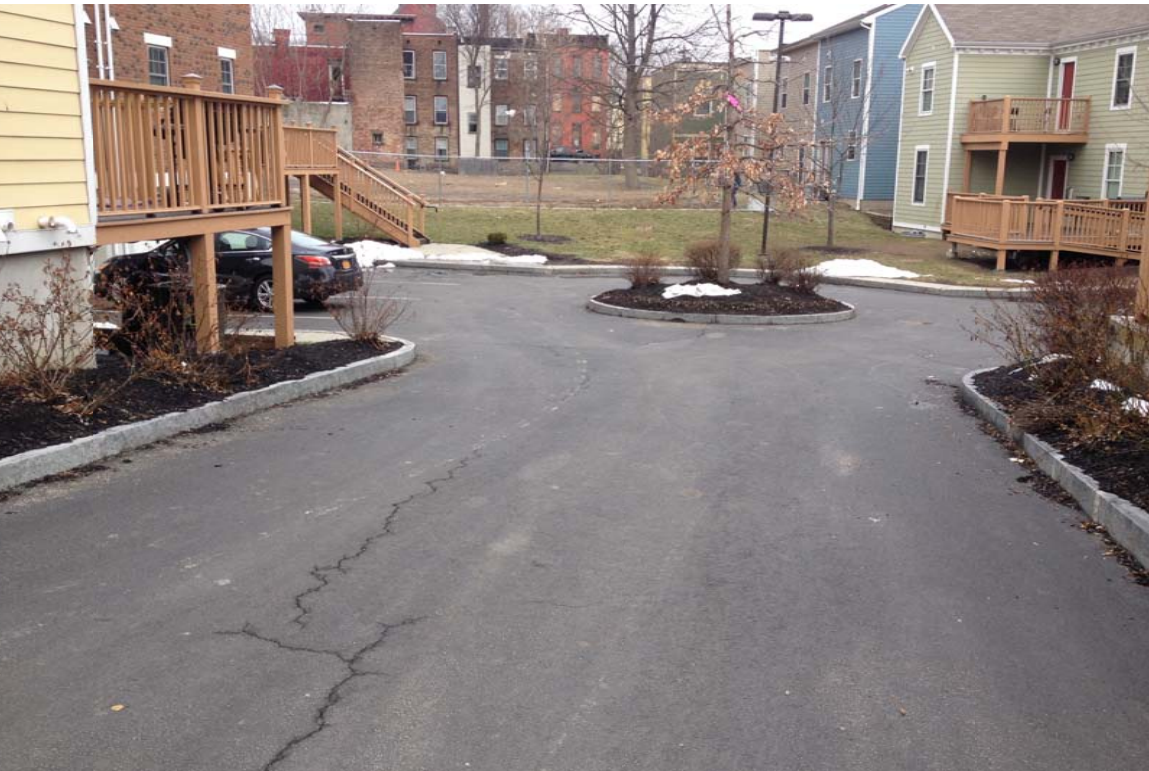
Minor cracking within the asphalt on the property
