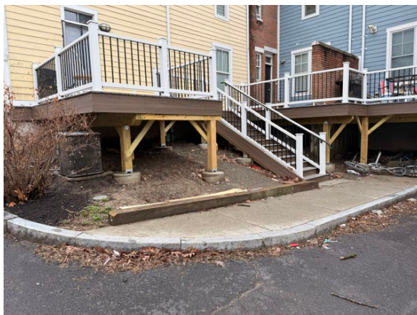
Photo #5 Slightly eroded areas underneath housing decking
