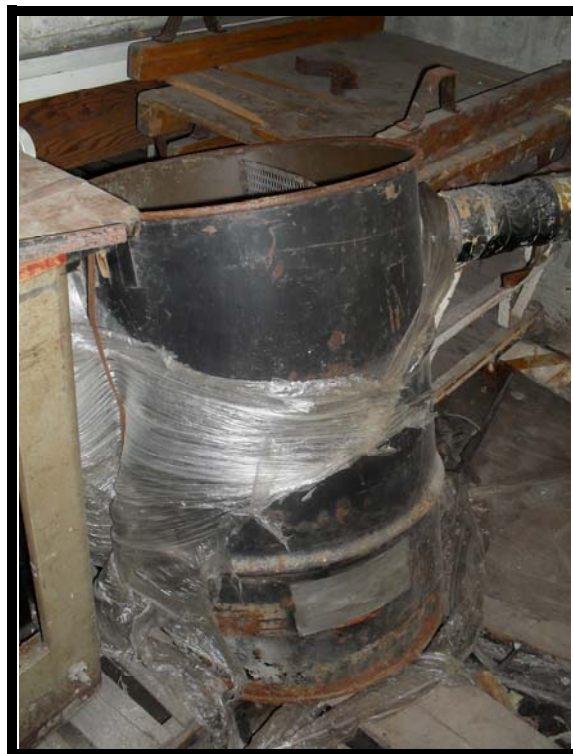
Building 1 Basement, Room 003 - Drum of Unknown Substance.
