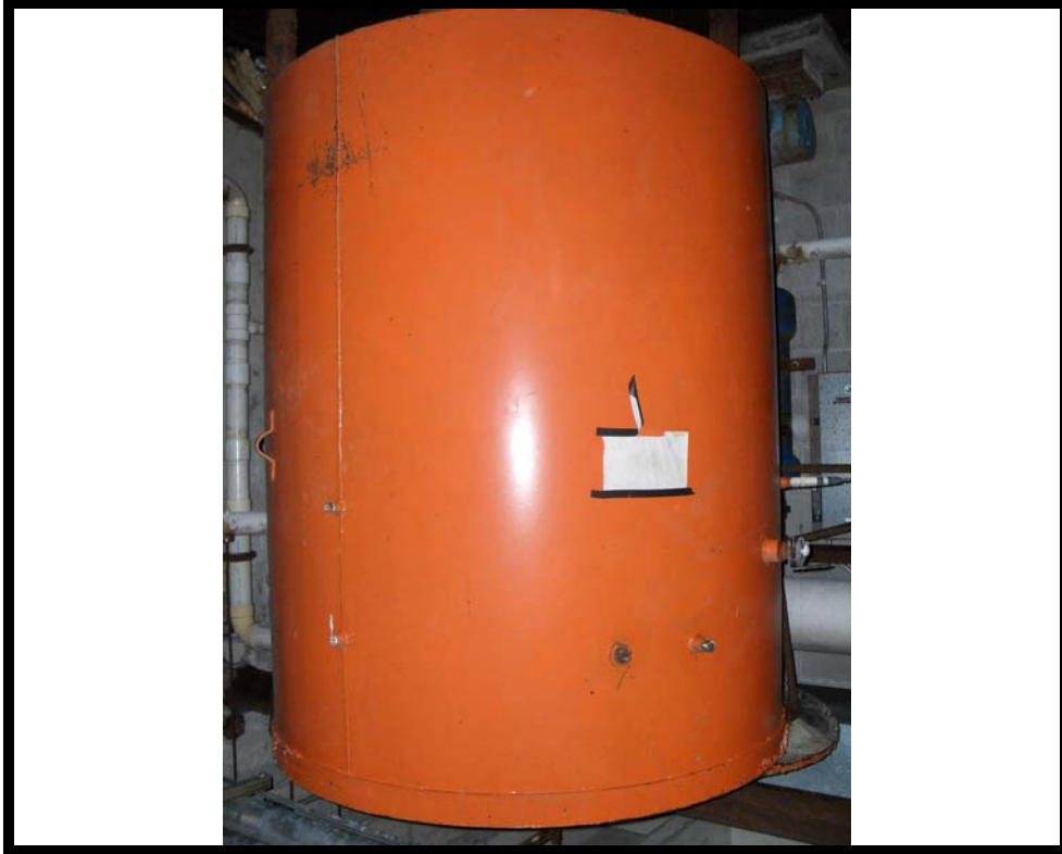
Building 1 Basement, Room 005 – Orange Steel Tank.
