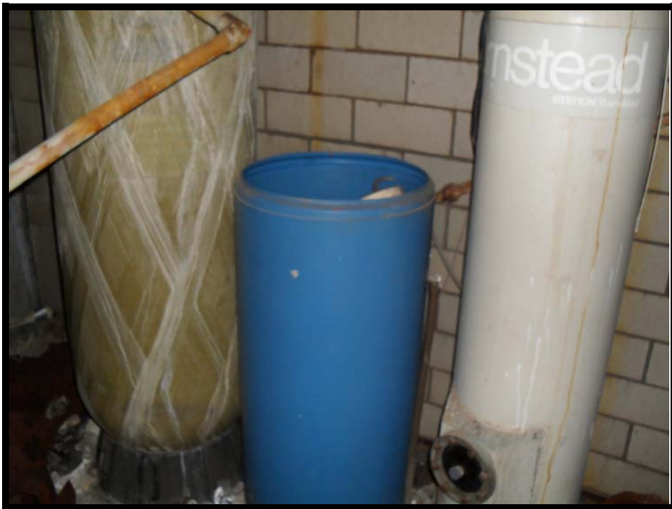
Building 11, Room B-2 – Deionization Tanks.
