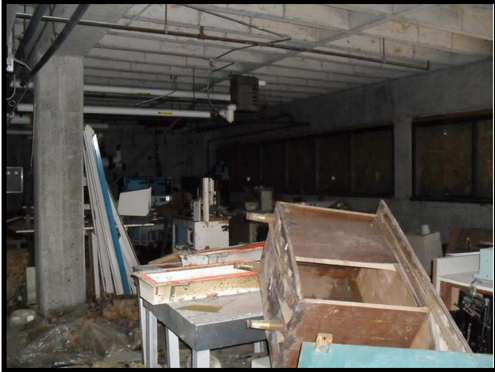
Building 1 Basement Room 004 – Miscellaneous Equipment.
