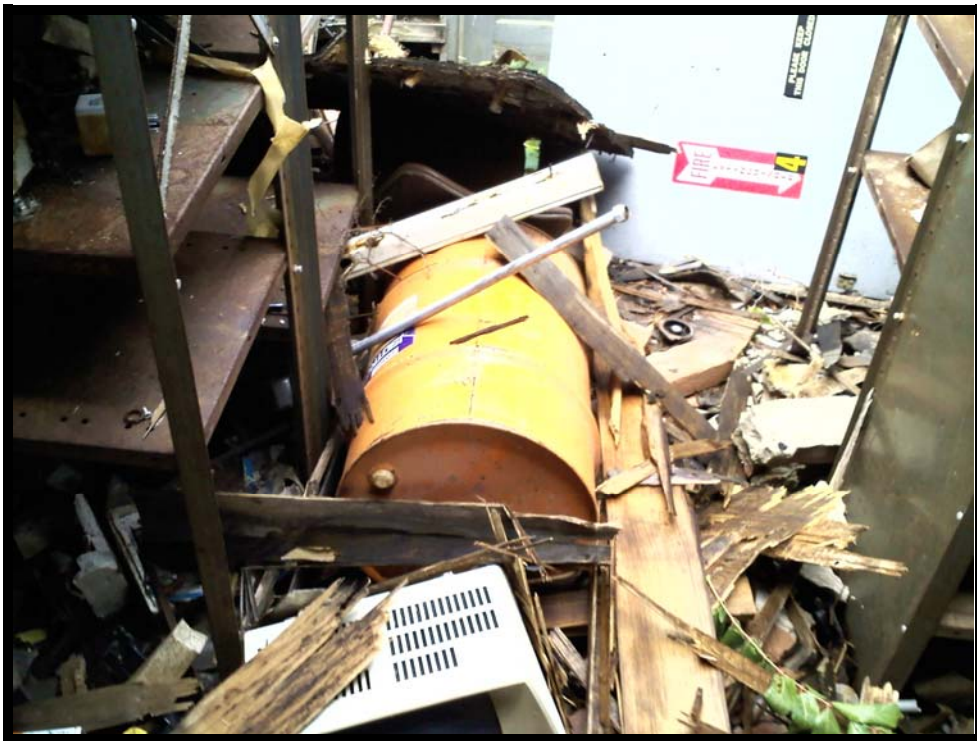
Building 4 Electrical Room – Debris and Trichlorofluoromethane Drum.
