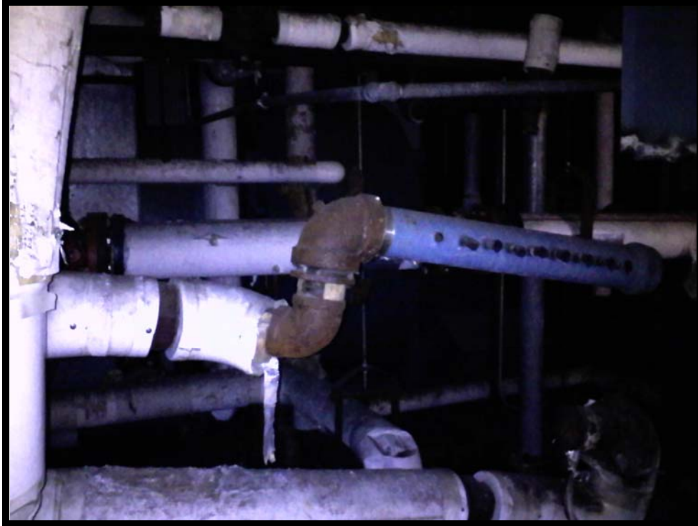
Building 9 Kathabar Conditioning System Piping.
