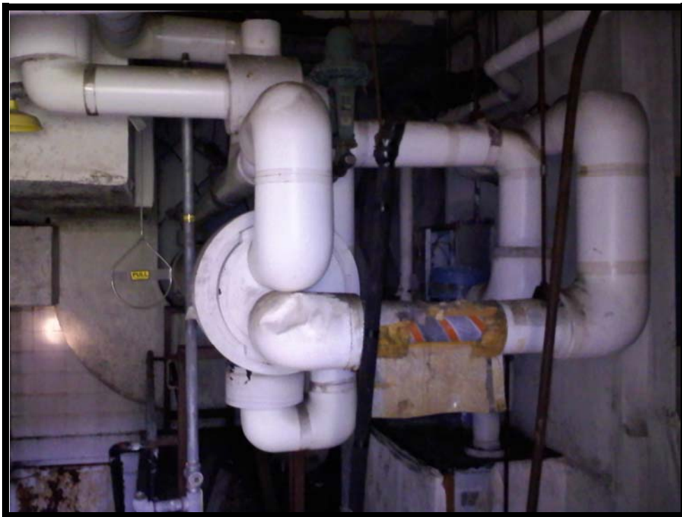
Building 17 Kathabar Conditioning System Piping.
