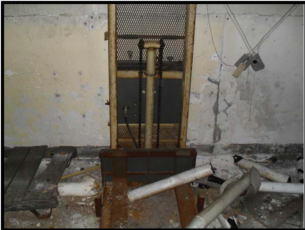
Building 2 Second Floor, Chill and Noodling Room – Single Piston Hydraulic Lift.
