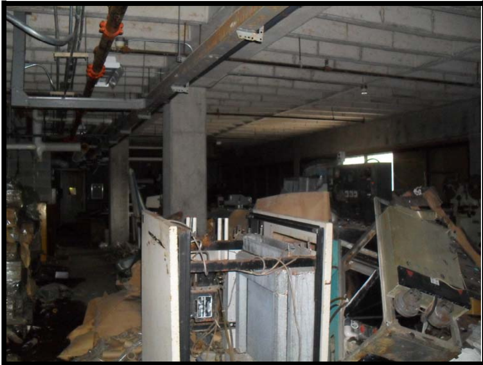
Building 1 Basement, Room 004 – Miscellaneous Equipment.
