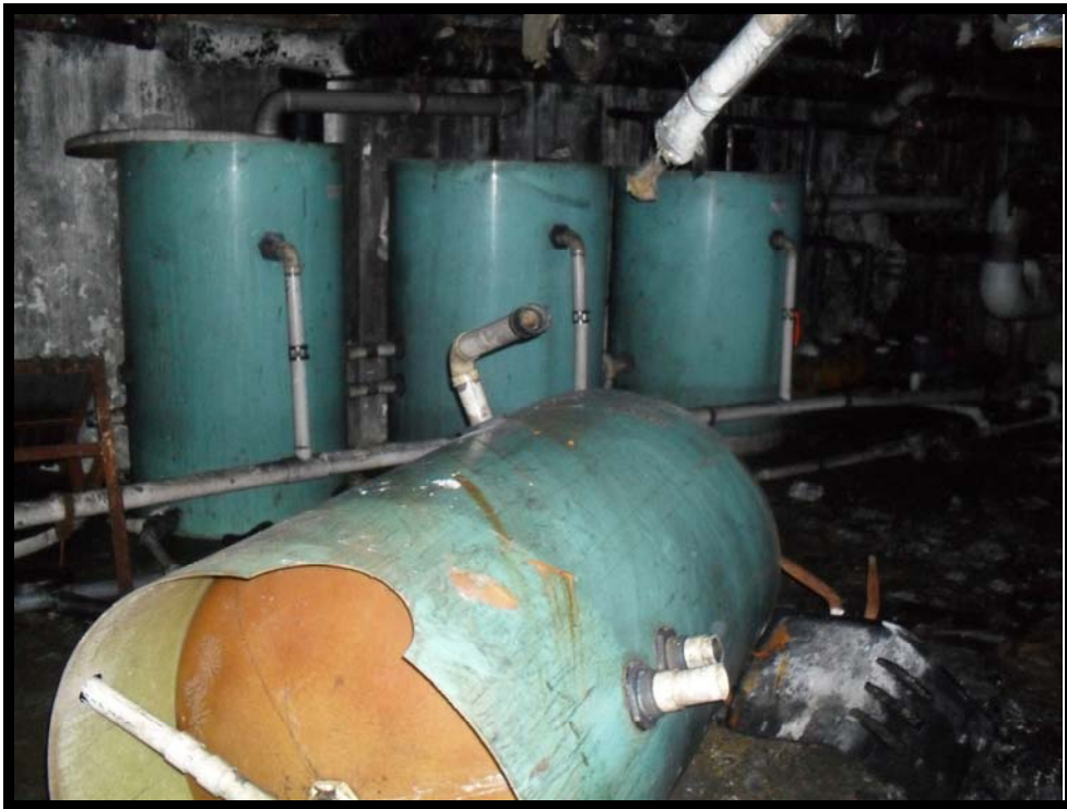
Building 2 Basement, Bulk Storage Room – Four 250-gallon Poly Tanks.
