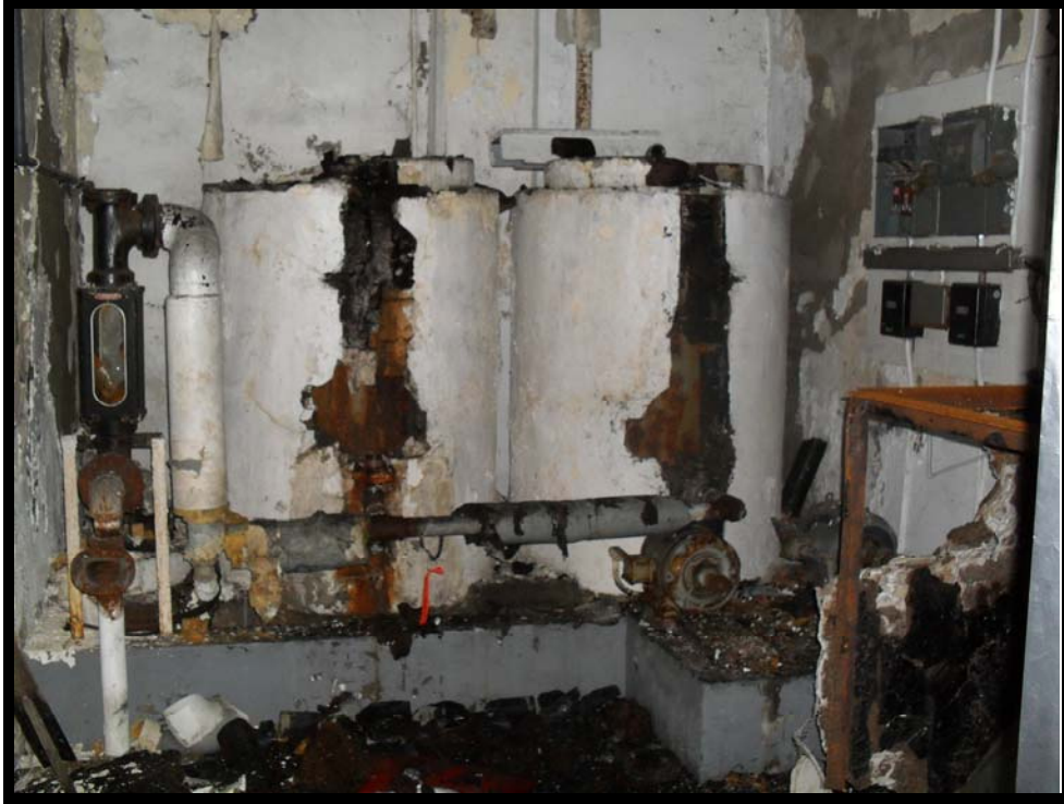
Building 2 First Floor, Room 111 – Two Tanks and Trough with Unknown Liquid.
