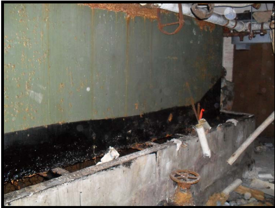
Building 2 Basement, Bulk Storage Room – Rectangular Tank and Trough.
