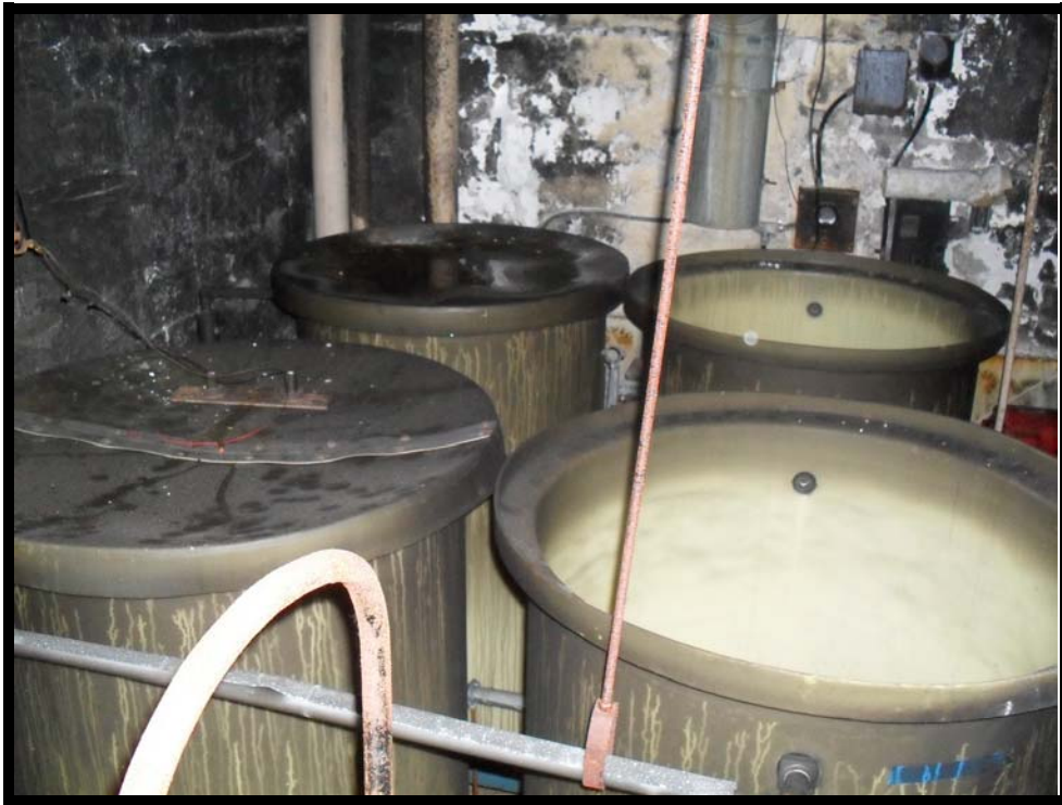
Building2 Fourth Floor – Still Room Poly Water Tanks.
