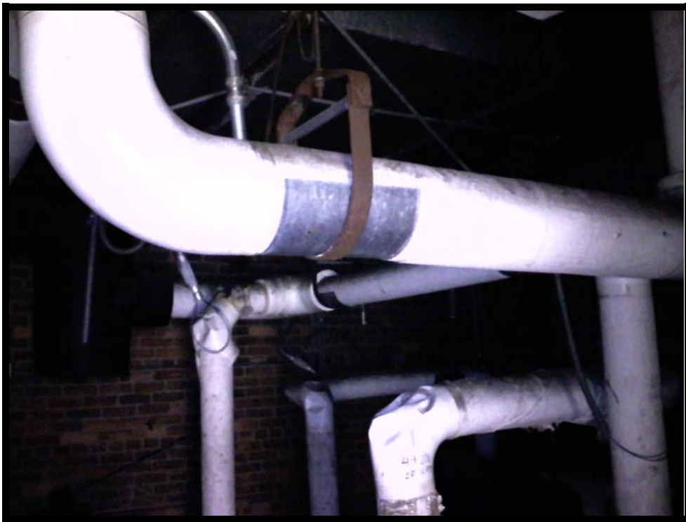
Building 9 Kathabar Conditioning System Piping.
