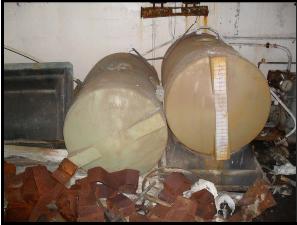
Building 11, Room B-2 – Deionization System Tanks.
