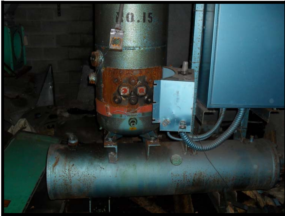
Building 1Basement, Room 005 – Water Chiller Pump and Freon Tank.
