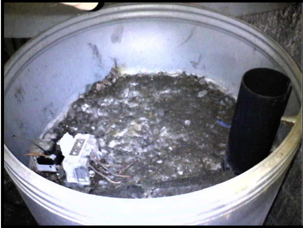
Building 5, Boiler House – White Drum with Foamy Unidentified Liquid.
