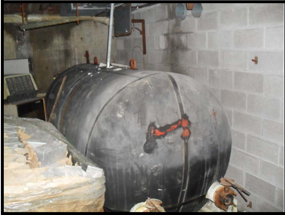
Building 1 Basement, Room 003 in Northeast Corner – Chill Water Tank.
