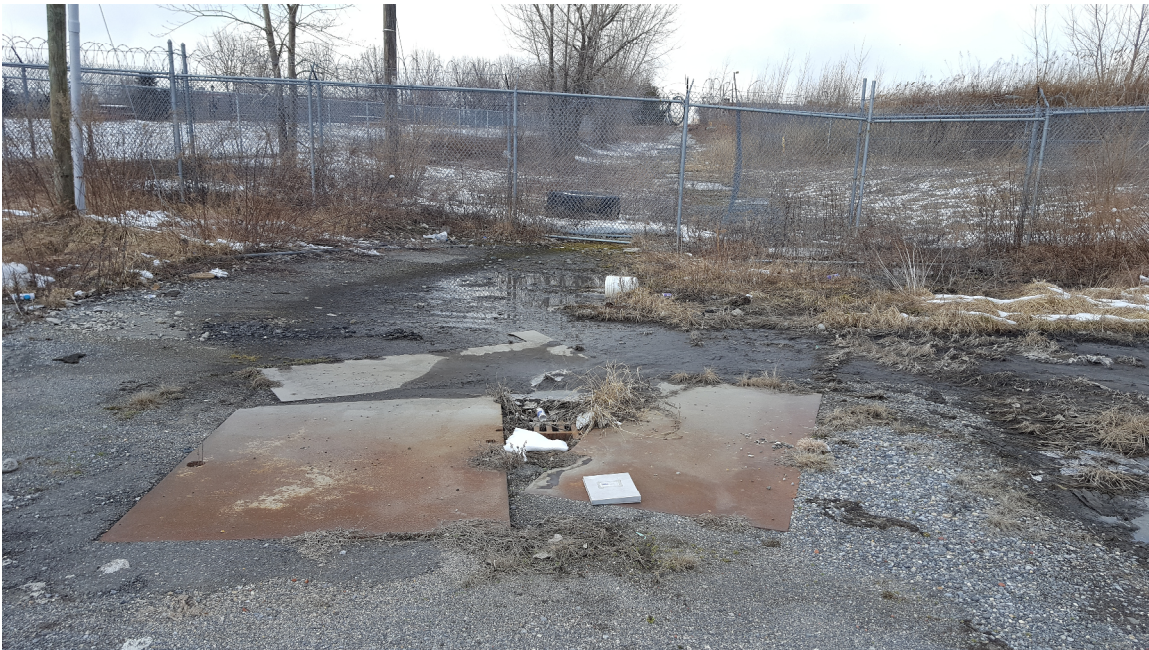
Photograph #12 – Stormwater catch basin in topographically low area near intersection of Barretto Street and Ryawa Avenue. Steel road plates may be covering area of subsidence. Barretto Street extending north beyond fence.
