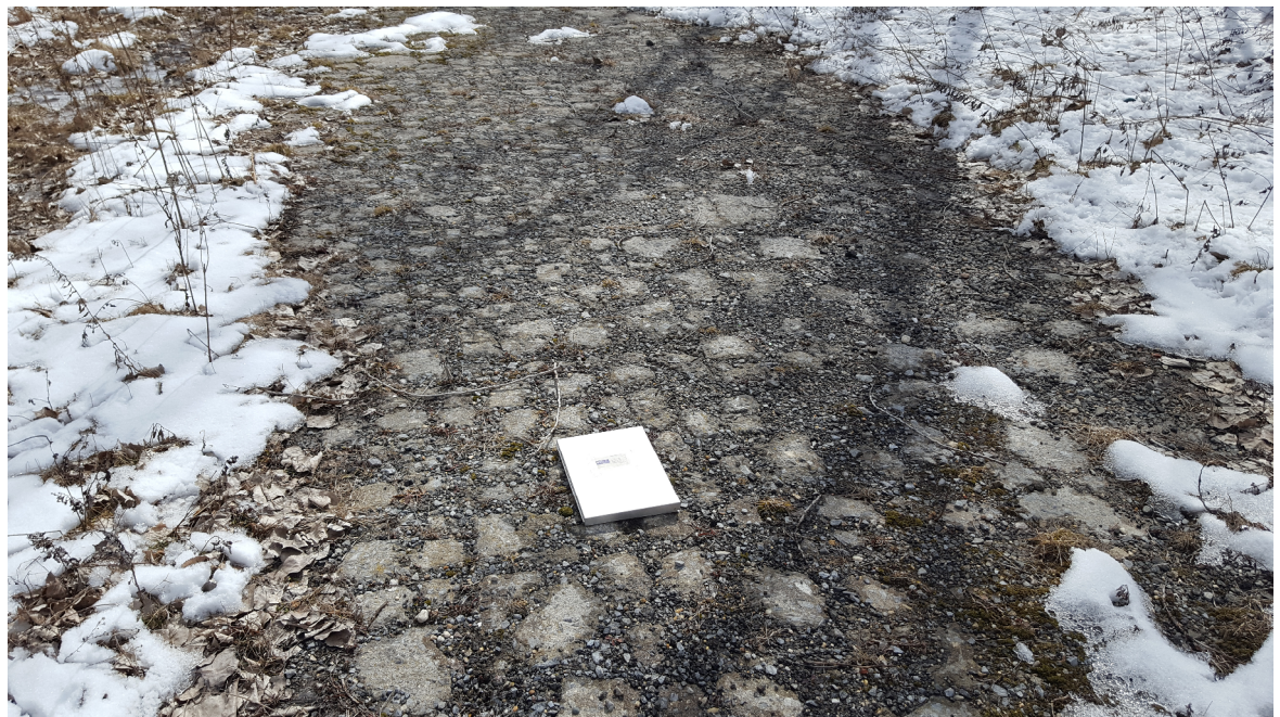
Photograph #4 – Deteriorated Barretto Street pavement.
