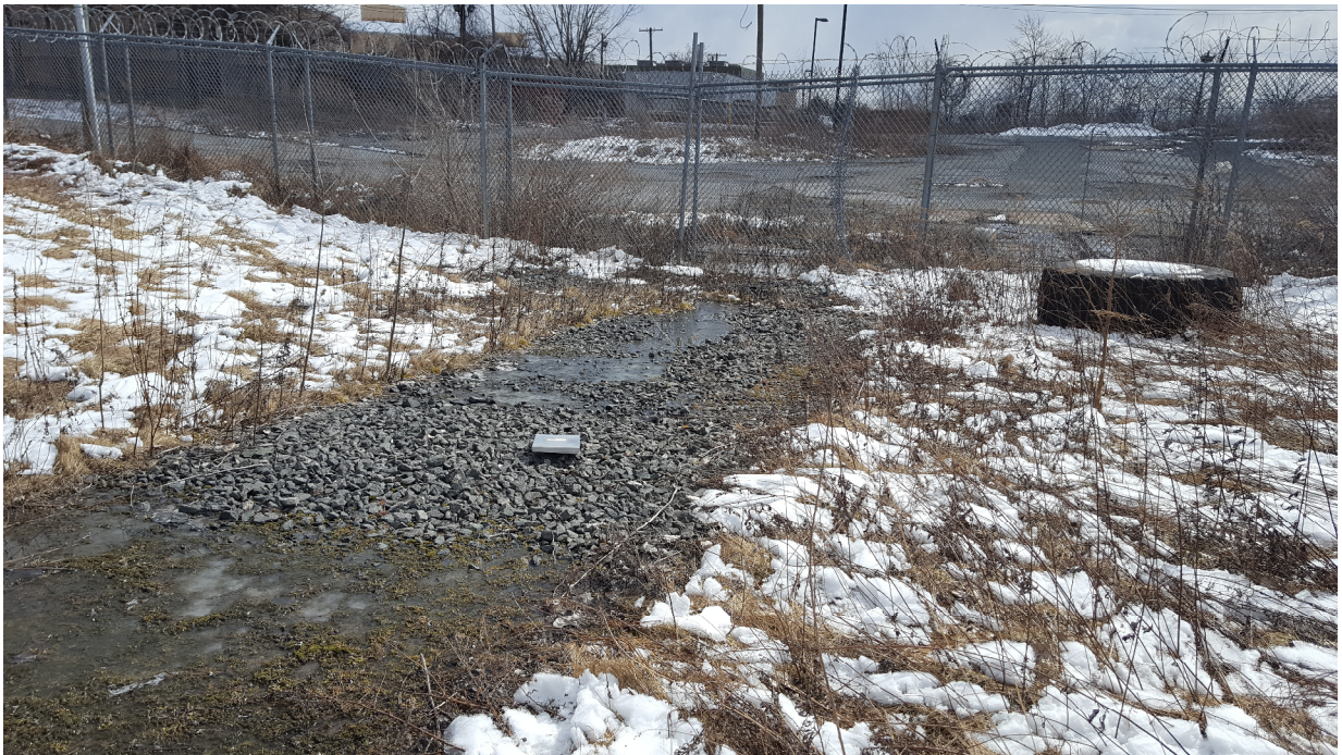
Photograph #5 – Stone and ponded water at south end of Barretto Street. Ryawa Avenue extending left to right beyond fence.
