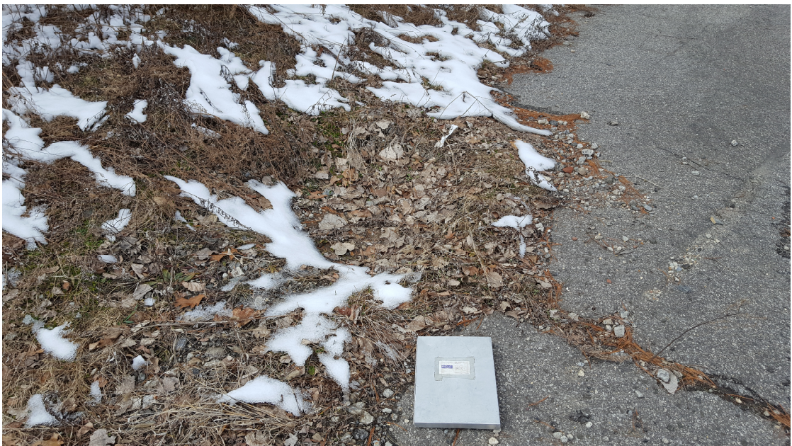
Photograph #2 – Surface depression (apparent subsidence) adjacent to Barretto Street pavement. Depression is approximately 2 feet diameter, 10 inches deep.
