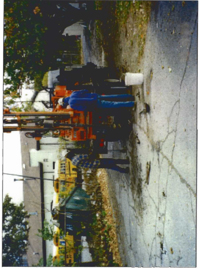
Drilling monitor well MW-4A on the northeastern corner of the parking lot.
