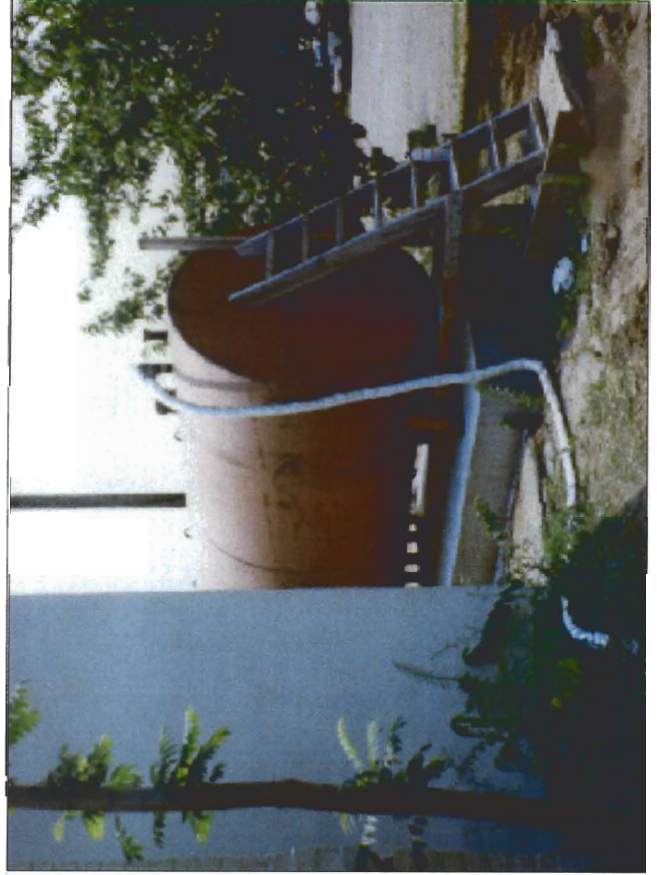
2,000-gallon fuel oil aboveground storage tank located on the western side of the building.
