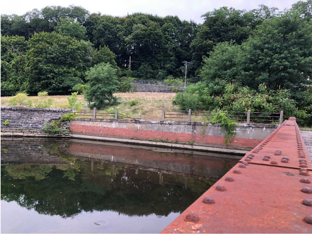
Photograph 5 – Damaged and missing railings on the retaining wall north of the creek
