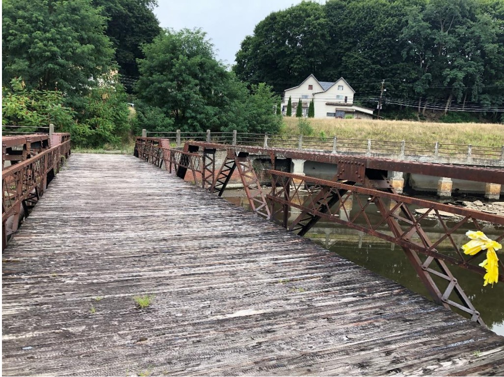
Photograph 4 – Missing side rails on the footbridge
