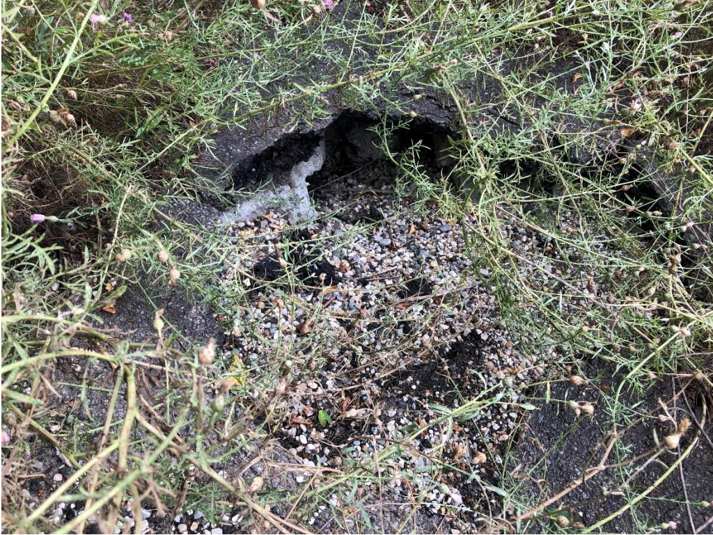
Photograph 2 – Pothole along the north side of the creek and retaining wall
