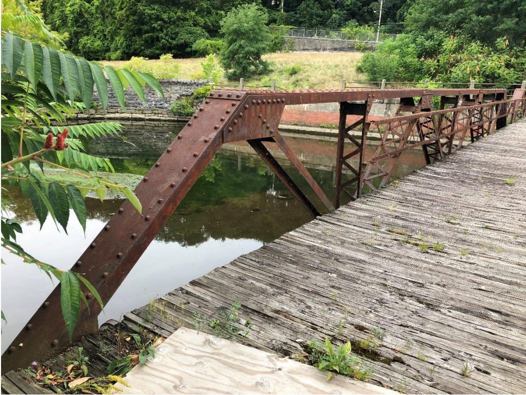
Photograph 3 – Missing side rails on the footbridge
