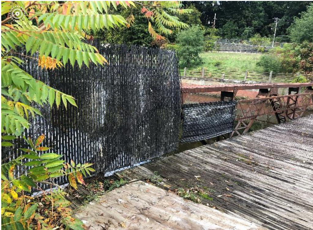
Photograph 3A – Repairs to the missing side rails on footbridge and missing railings on the retaining wall north of the creek
