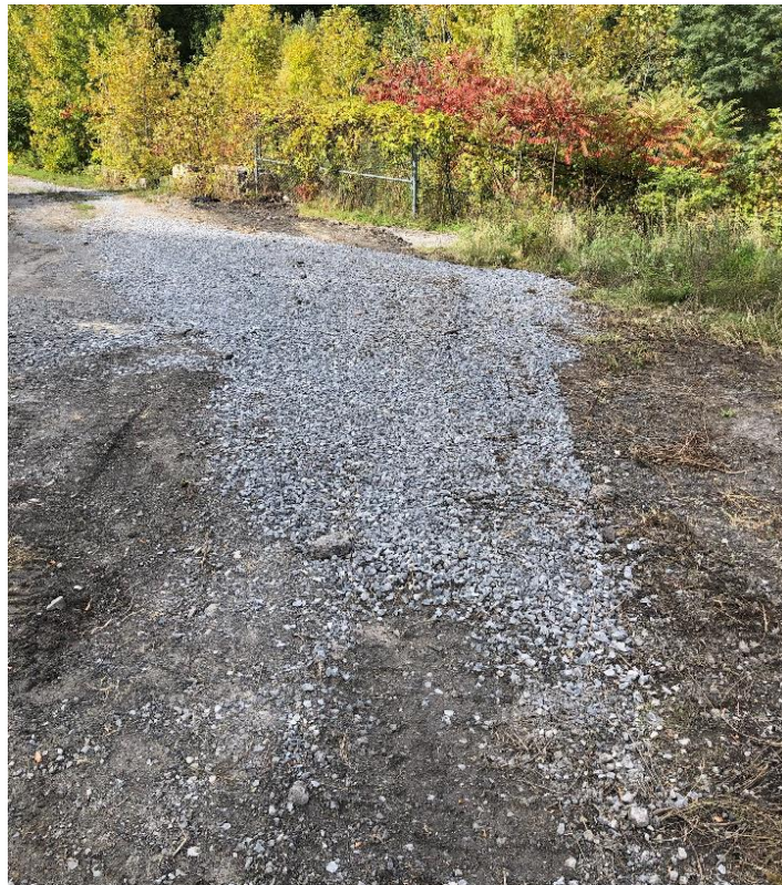
Photograph 1A – Repairs to the settling of the former foundation north of the existing building
