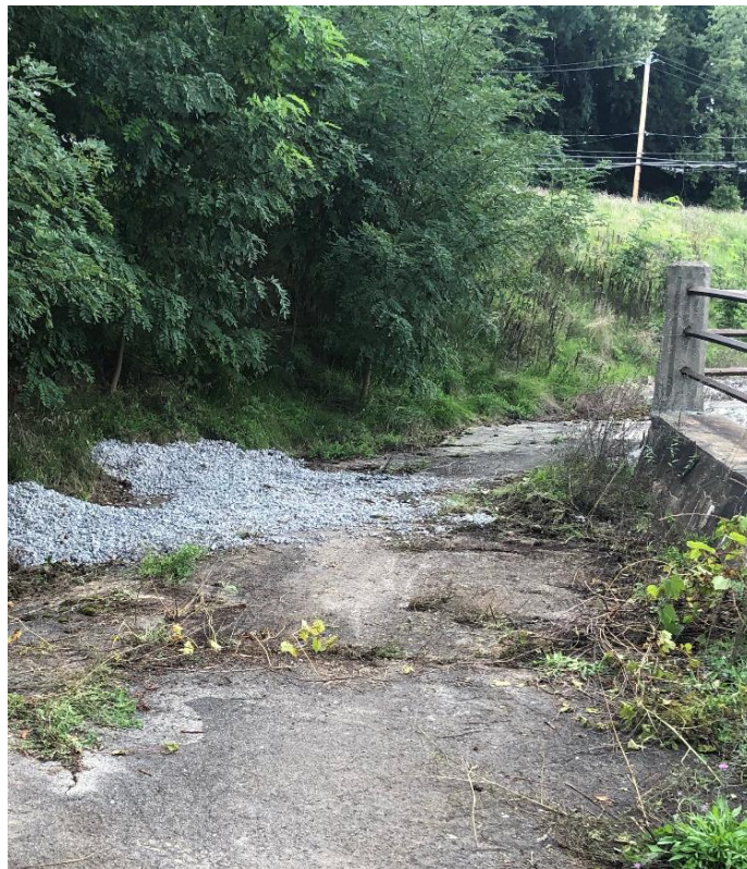
Photograph 2A – Pothole repairs along the north side of the creek and retaining wall
