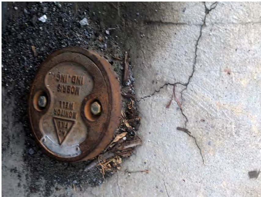
8. MW-3 at southeastern side of paved parking area (note: top portion of PVC well-casing is cracked)
