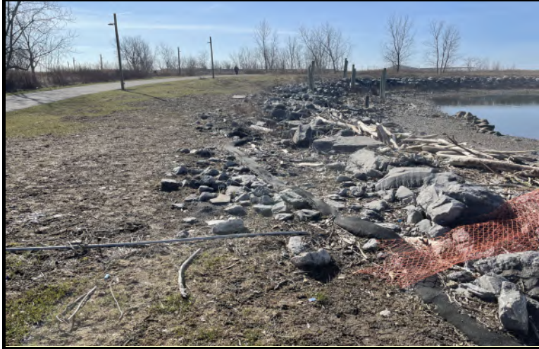
Photo 24: Repairs at Bell Slip. Vegetation required to be established.
