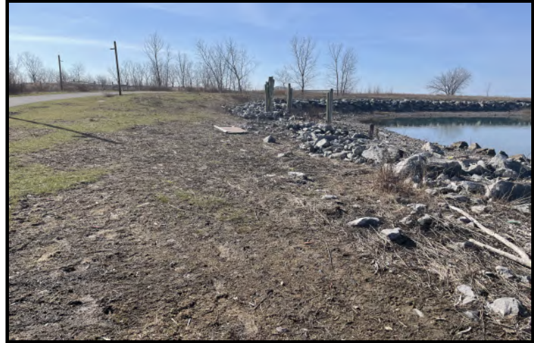
Photo 23: Repairs at Bell Slip. Vegetation required to be established.
