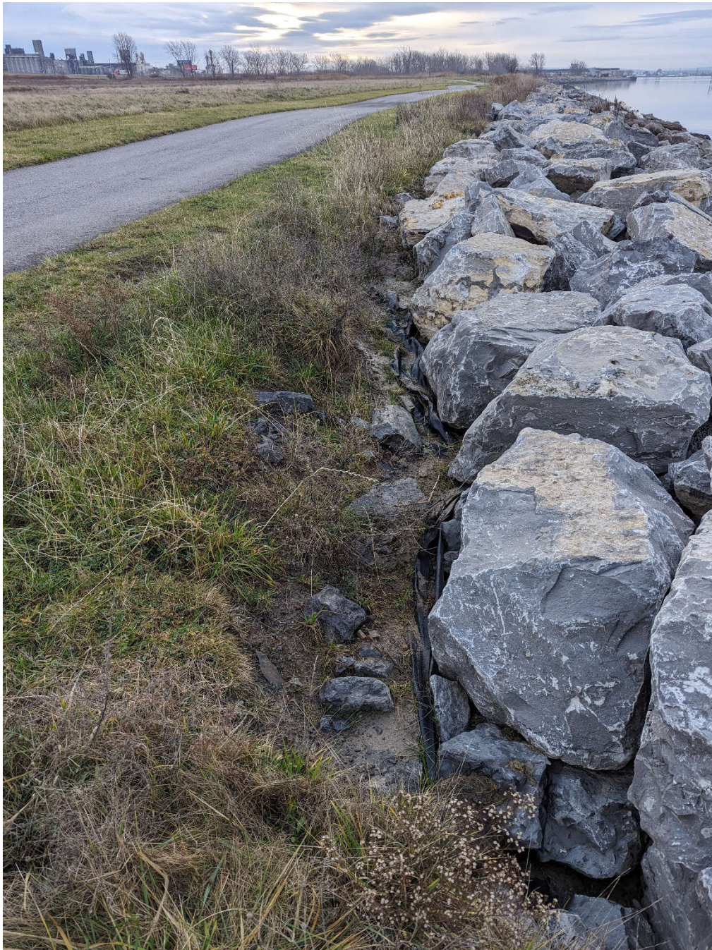
1.) View of minor erosion at the top of the stone revetment along the northern portion of the Pathway.
