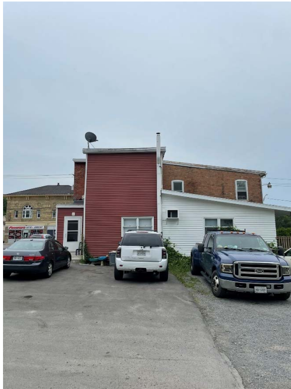
2626 Main St SSDS exterior piping – looking south
