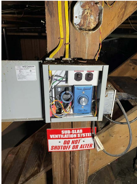
2626 Main St SSDS control box in basement
