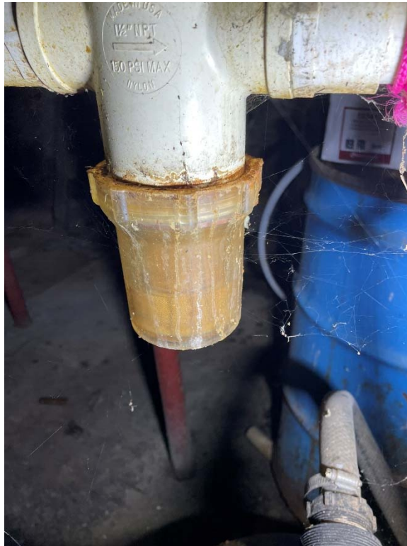
2626 Main St filter on basement sump discharge in front of carbon treatment system
