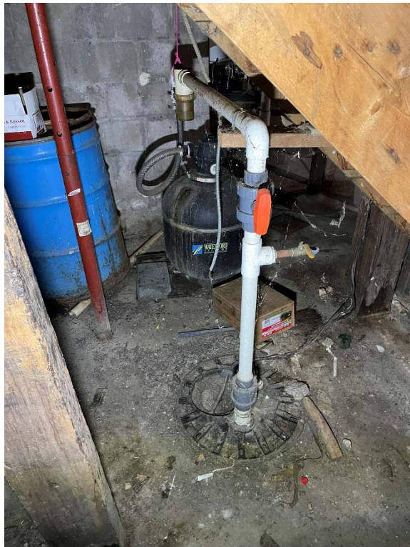
2626 Main St sealed and vented basement sump with discharge connected to carbon treatment system
