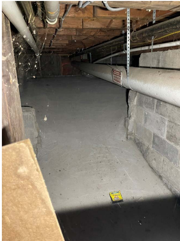
2626 Main St SSDS piping and labeling in basement
