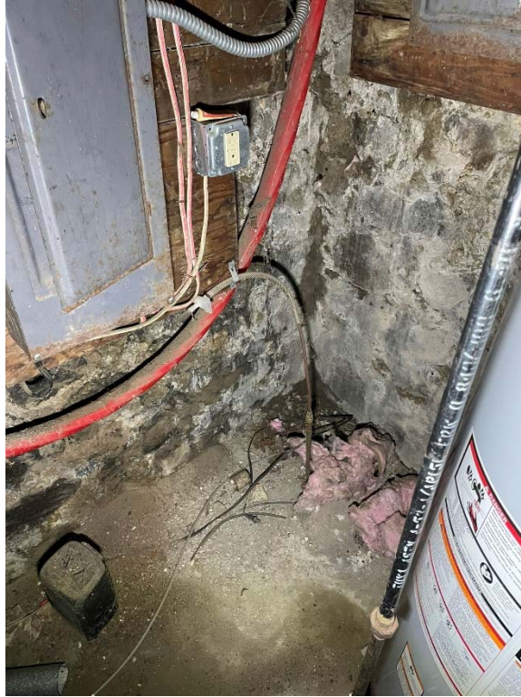
2626 Main St SSDS Monitoring Pt #1 in basement
