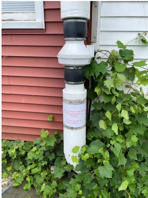
2626 Main St SSDS exterior fan and piping with new labeling – looking south
