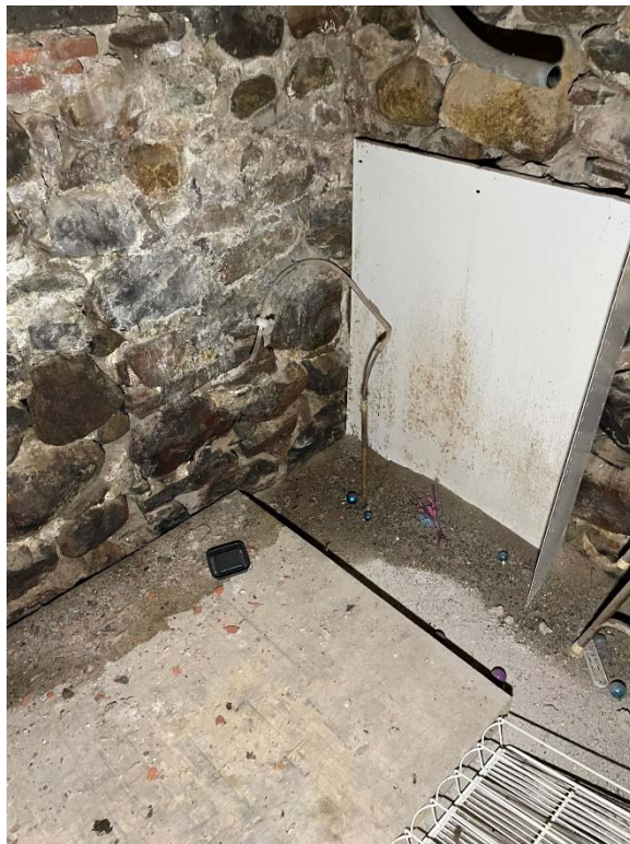
2626 Main St SSDS Monitoring Pt #2 in basement
