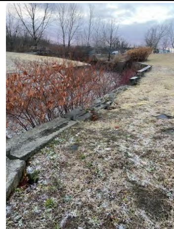
Multiple small holes located near the west retaining wall, southeast of MW-6 Photographed December 2023
