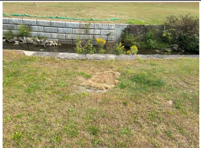
View of repaired animal burrow west of Cayadutta Creek
