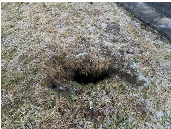
Hole located near the west retaining wall near MW-6, looking north Photographed December 2023
