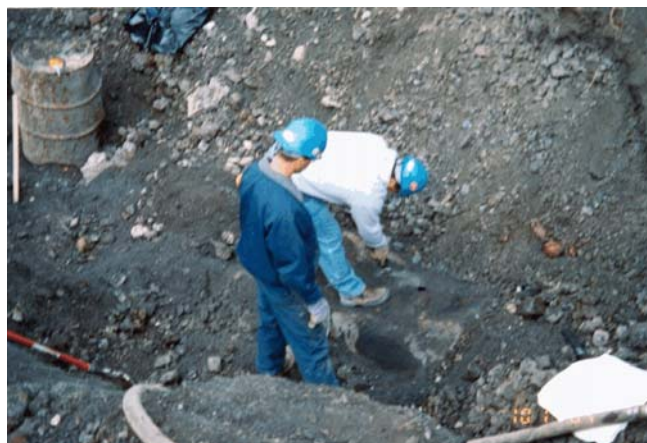
Buried Drum and Tank
