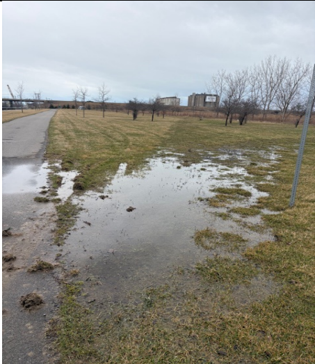
11. North side looking west at field and asphalt path, some seasonal pooling and mild rutting
