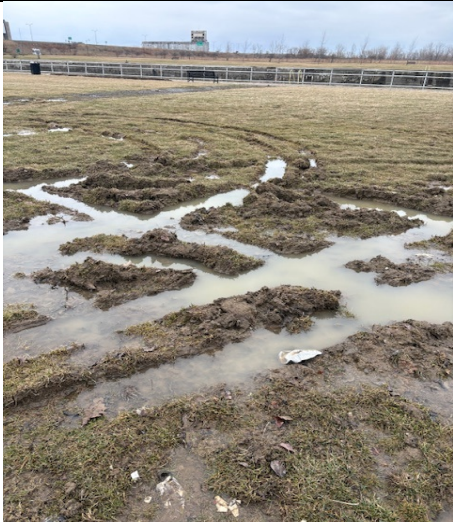
22. South side looking northwest at rutting
