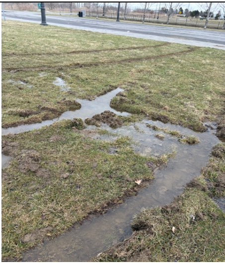
20. South side looking south at rutting
