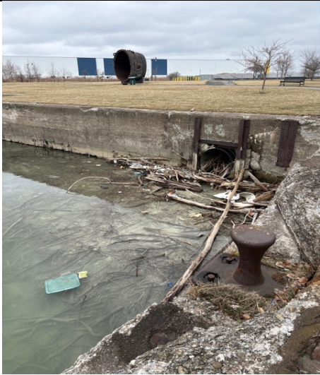
34. South side looking east at end of canal, canal wall in good condition
