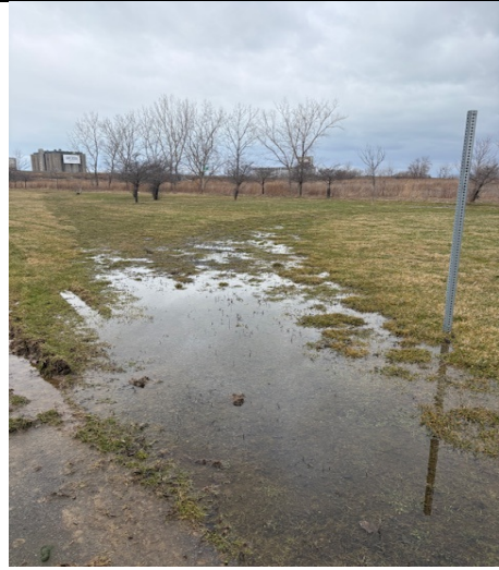
12. North side looking northwest at field, some seasonal pooling and mild rutting
