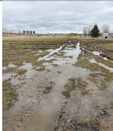
25. South side looking east at rutting
