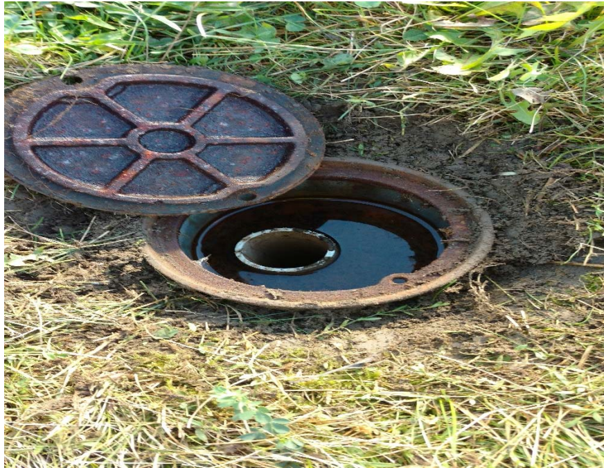
Monitoring Well MW-3 (water in curb box and missing j-plug).
