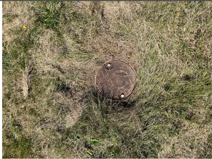
View of typical monitoring well
