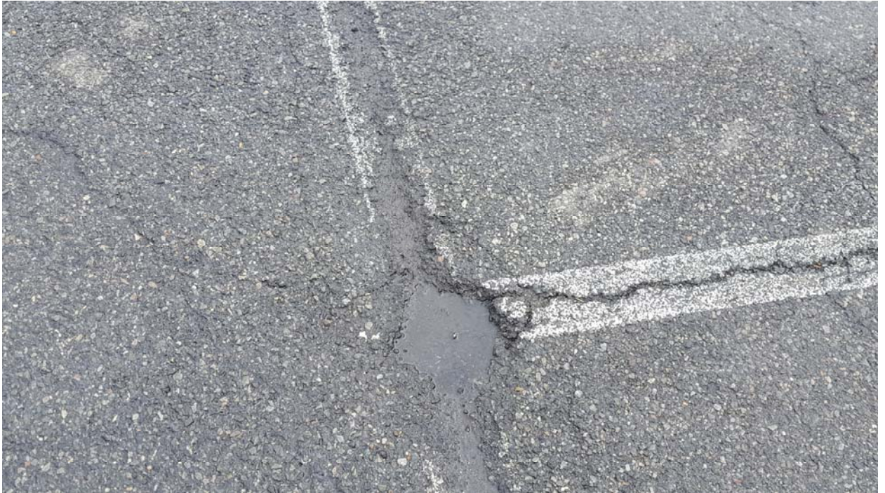
PHOTO 11: ASPHALT SURFACE - (SMALL SECTION MISSING - ASPHALT LAYER UNDER THIS)
