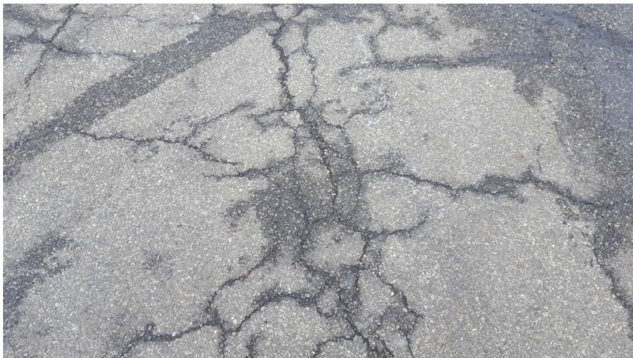
PHOTO 8: ASPHALT SURFACE CRACKS
