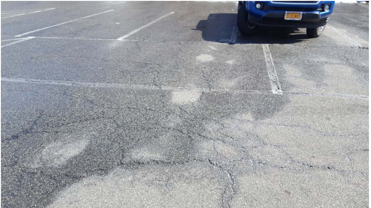
PHOTO 9: ASPHALT SURFACE CRACKS
