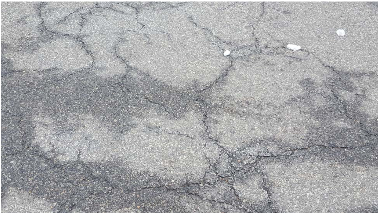
PHOTO 10: ASPHALT SURFACE CRACKS
