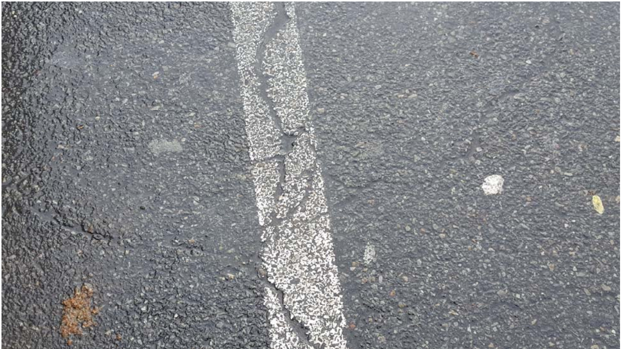
PHOTO 12: ASPHALT SURFACE CRACKS
