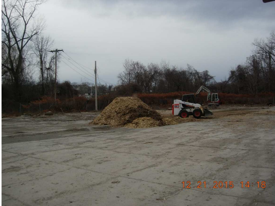
Chip pile remaining on concrete slab
