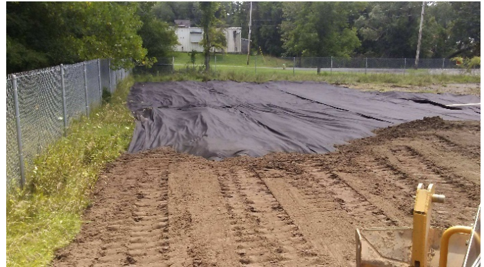
Demarcation layer placed beneath topsoil and on top of existing grade in the NE corner of the site
