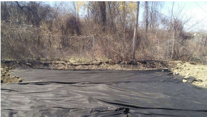
Demarcation layer placed along the southwest Perimeter at the excavation and removal area
