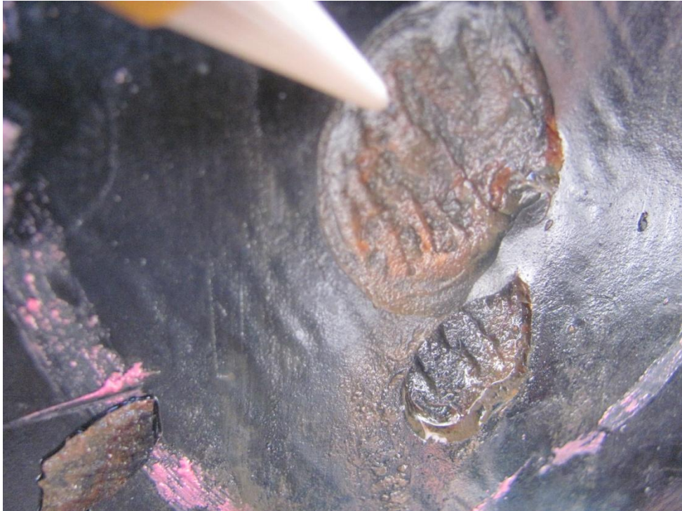
Photo 10 – Coating delamination with slight metal loss of approximately .005”.
