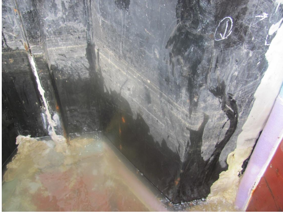
Photo 3 – North side of excavation. Note various rust spots with (black) coating.
