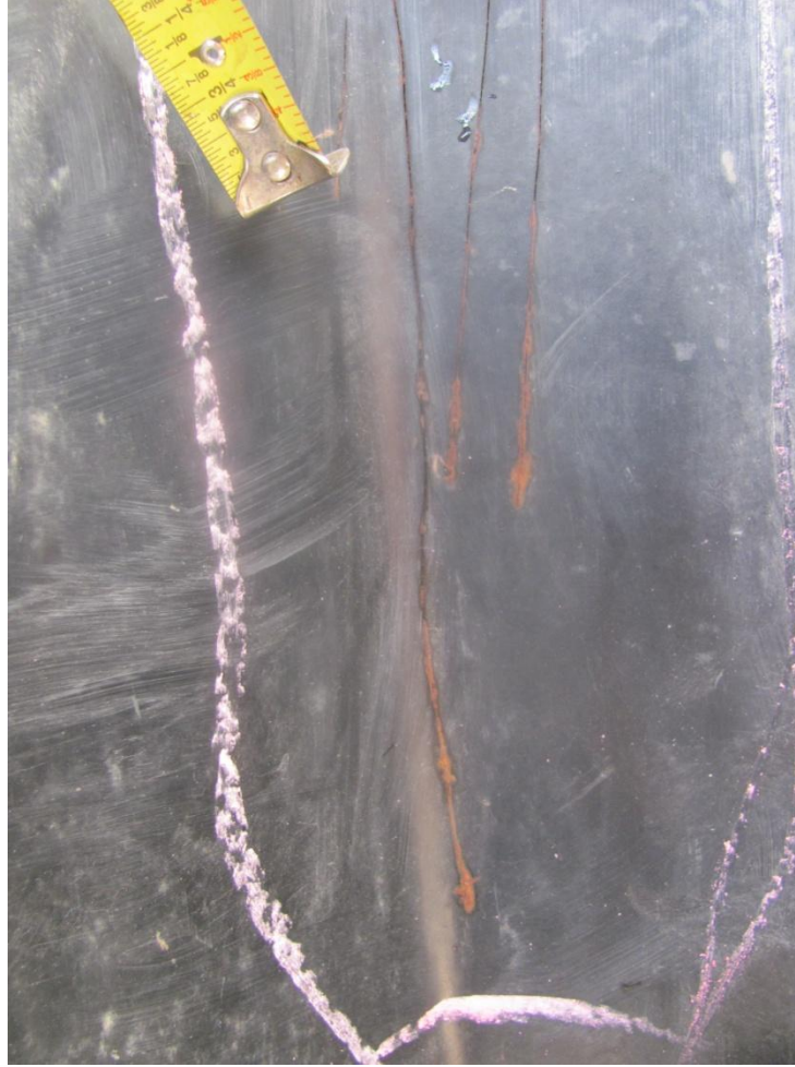
Photo 8 – Close-up of previous photo of vertical corner coating cracks with rust bleed.
