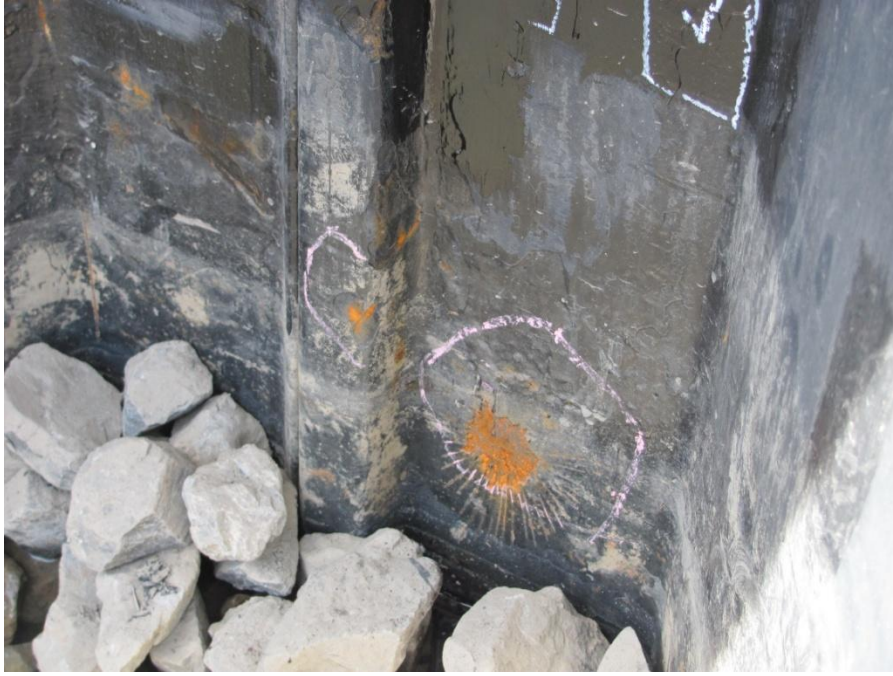
Photo 3 – Limited, failed/damaged areas requiring remedial coating work.
