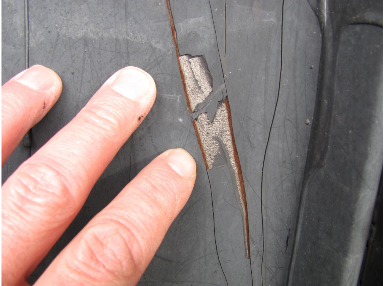
Photo 3 – Typical vertical coating cracks. Note through-crack rust.
