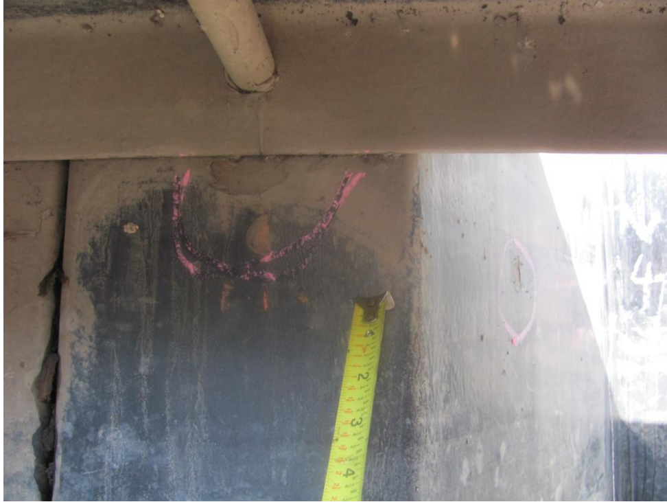
Photo 9 – Coating delamination on 1P176 adjacent to horizontal bracing (whaler).
