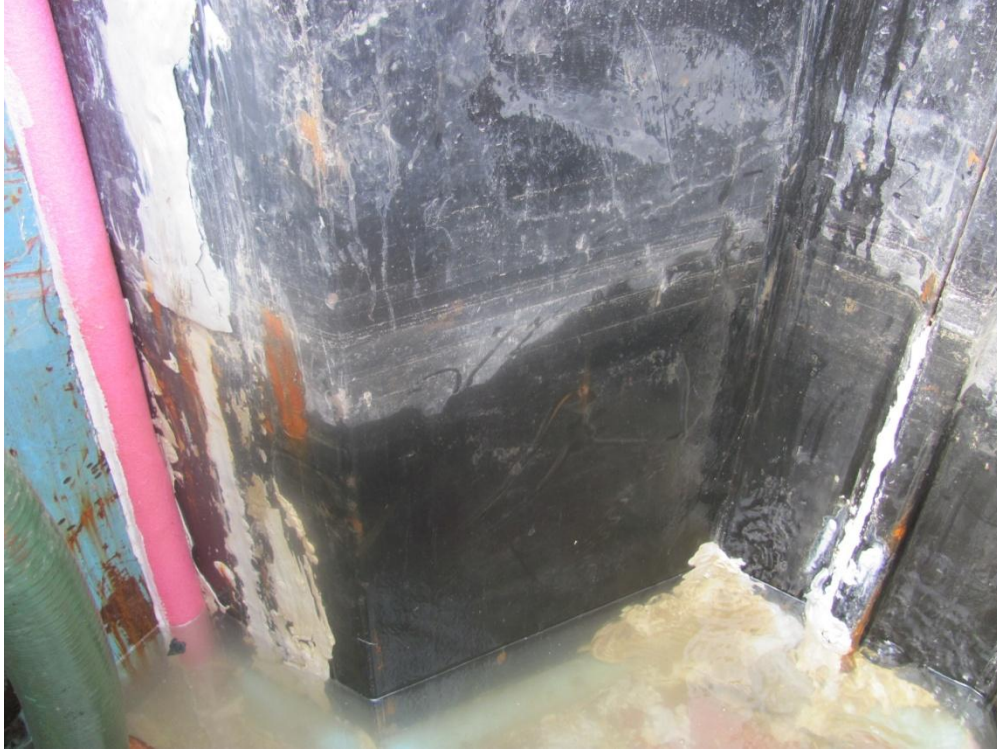
Photo 1 – South side of excavation. Note various rust spots with black coating section.
