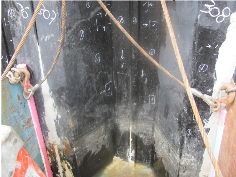
Photo 4 – Excavation overview. Note above grade coating repairs as indicated by white markings.
