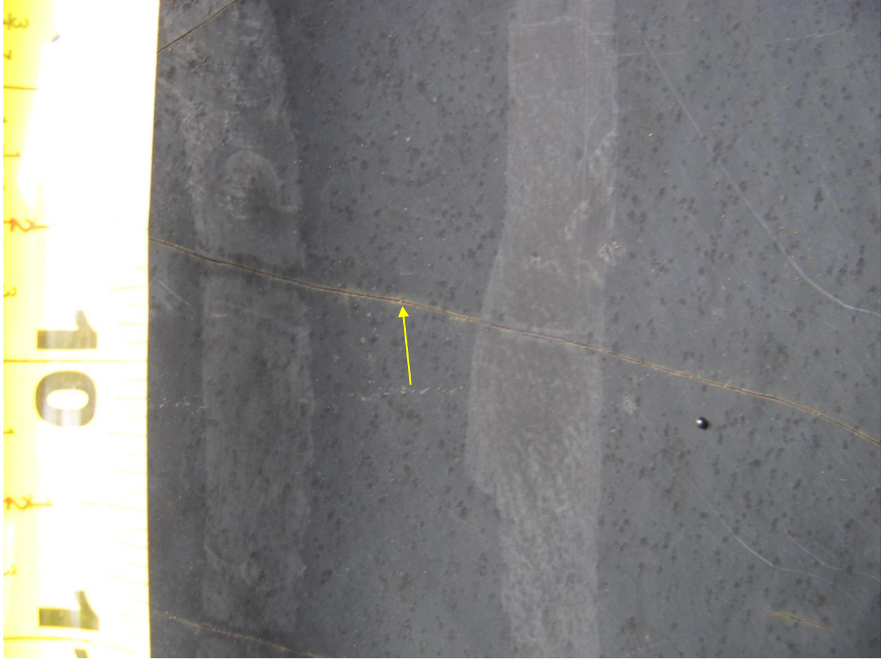
Photo 5 – Typical horizontal coating crack.
