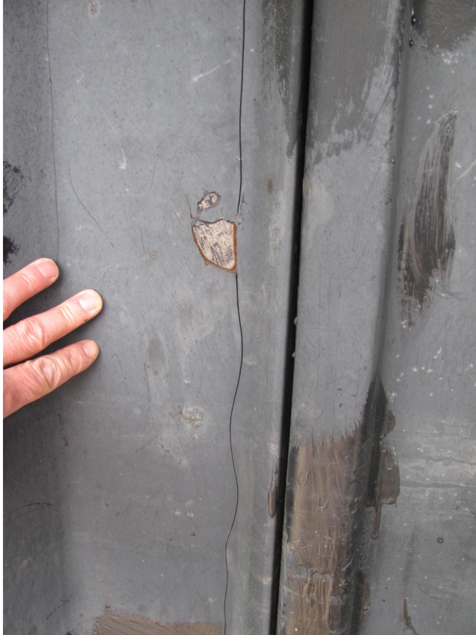
Photo 4 – Typical vertical coating crack associated with interlocks.
