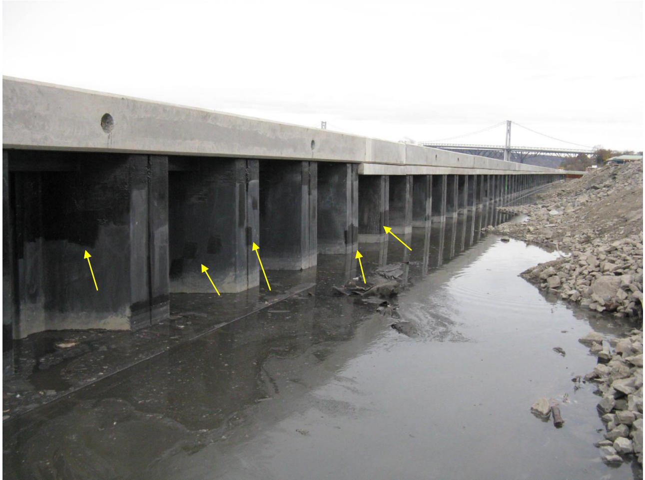
Photo 1 – Zone 1 looking north. Note numerous coating touch-up areas.
