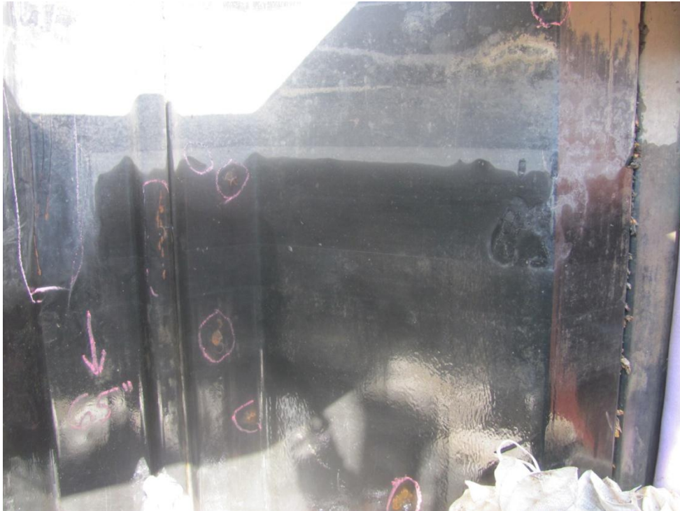
Photo 7 – Note vertical corner cracks (upper left), knuckle crack and various 1P176 coating failures with rust. See Photo 8 for crack area close-up.
