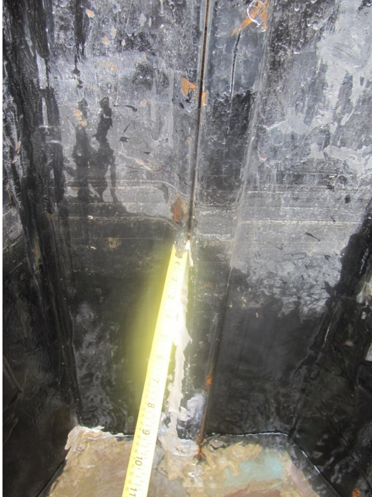
Photo 2 – Seam between Sheet Piles 307 and 308 at center of the excavated zone. Note various rust spots.
