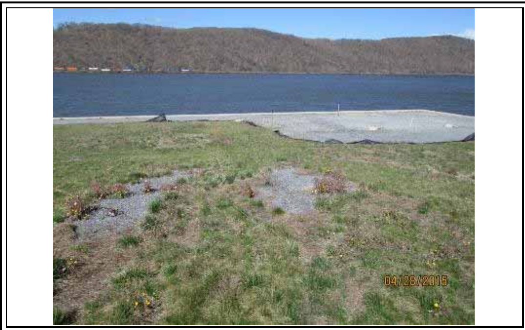
Photo 22 – Looking northwest; northern portion of Zone 1; previously repaired areas of scour.
