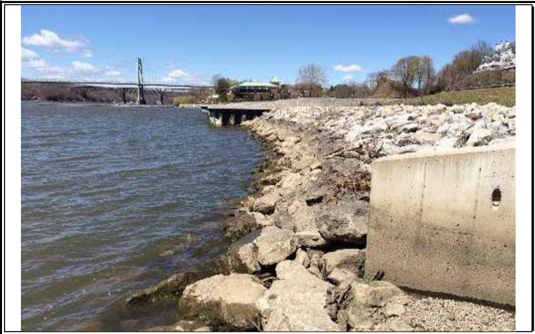
Photo 6 – Looking north; northernmost portion of Zone 2 riprap revetment; southern end of Zone 3 bulkhead.
