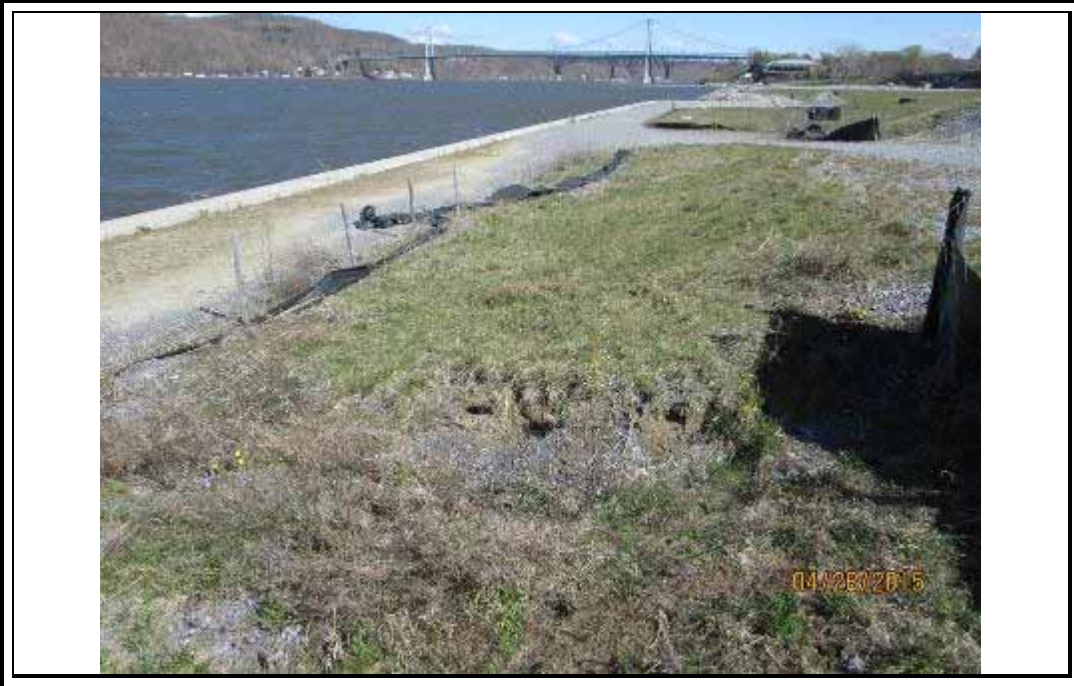
Photo 21 – Looking northwest; scour near southern end of Zone 1.
