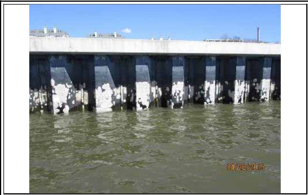
Photo 65 – Zone 3 bulkhead. (Note: Leaking interlock between sheets 75 and 77)
