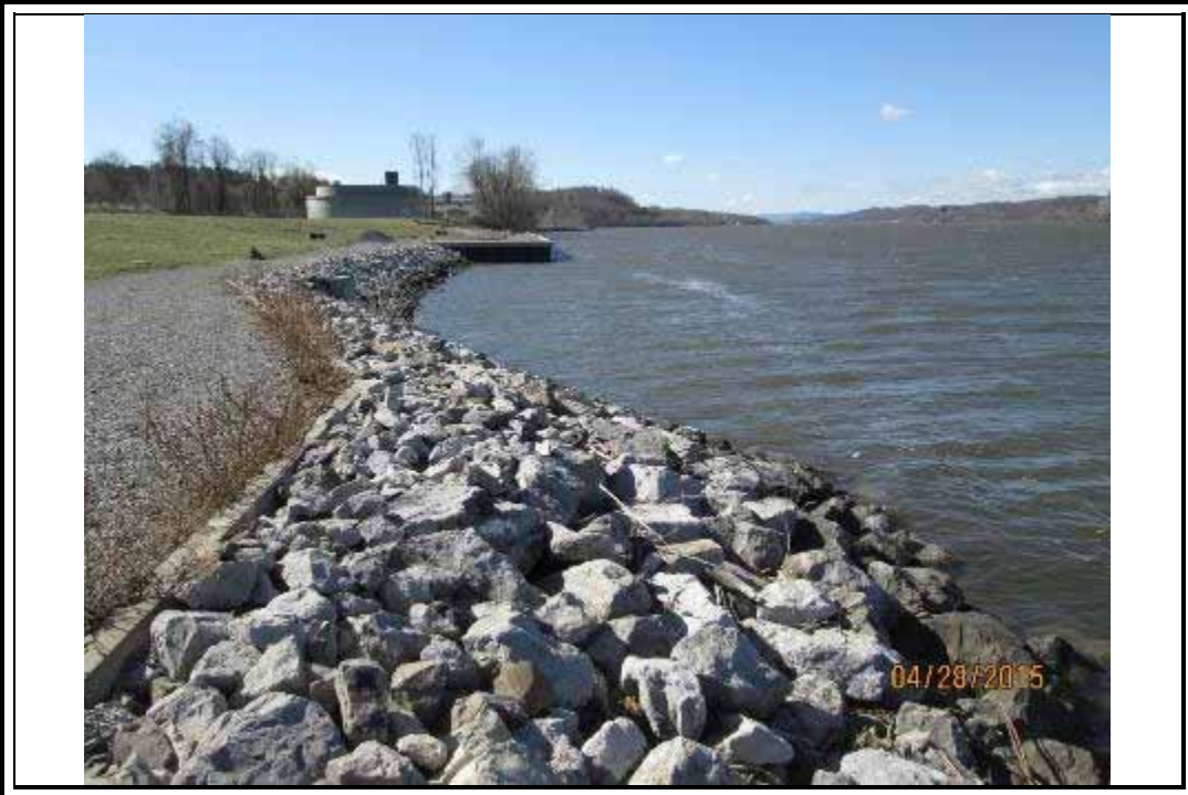
Photo 11 – Looking south; southernmost portion of Zone 2 riprap Revetment; northern end of Zone 1 bulkhead.
