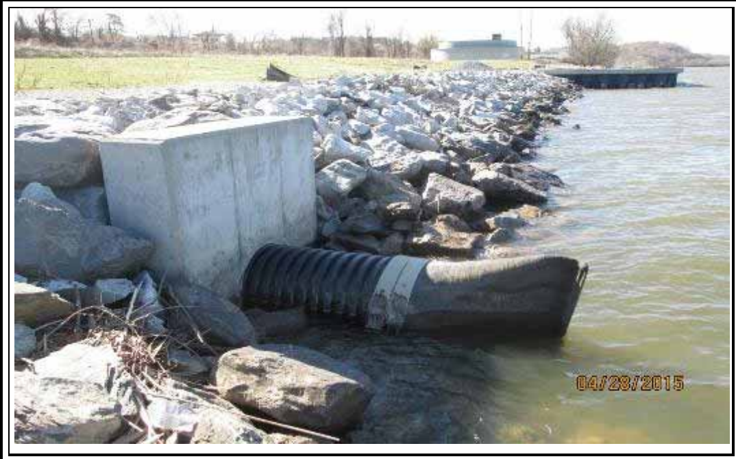
Photo 12 – Looking south, southeast; outfall/ drainage structure within southern portion of Zone 2 riprap revetment.
