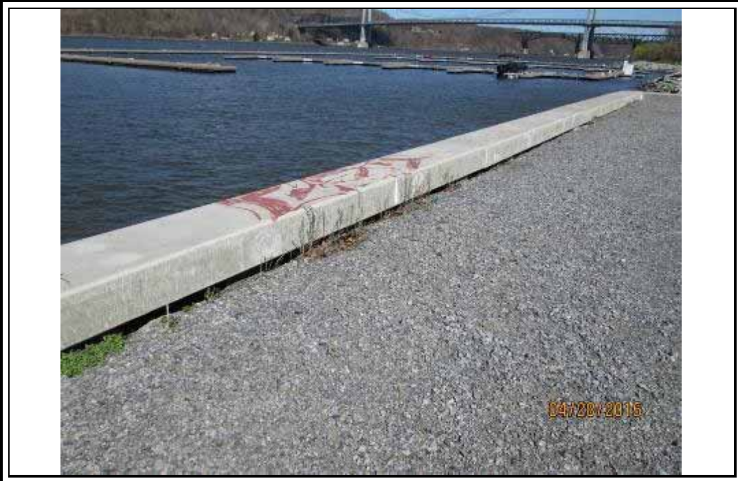
Photo 27 – Looking northwest; northern portion of Zone 3 bulkhead; note settlement of fill behind sheet piles, beneath concrete cap.
