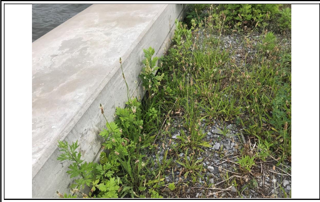
Photograph 19. Gap between the soil cover system and the bulkhead/concrete cap on the bulkhead observed in Zone 3.
