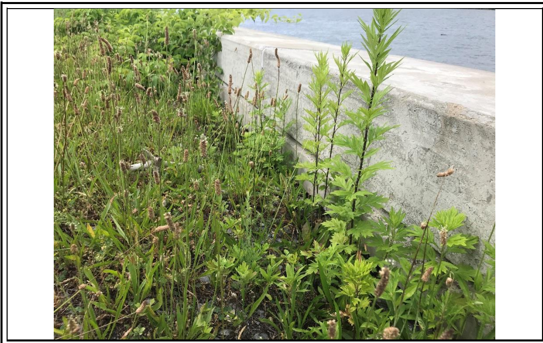
Photograph 20. Gap between the soil cover system and the bulkhead/concrete cap on the bulkhead observed in Zone 3.
