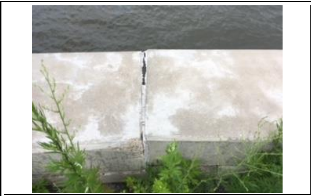
Photograph 10. Significant gap in the precast concrete cap on top of the bulkhead that is angled toward the river.
