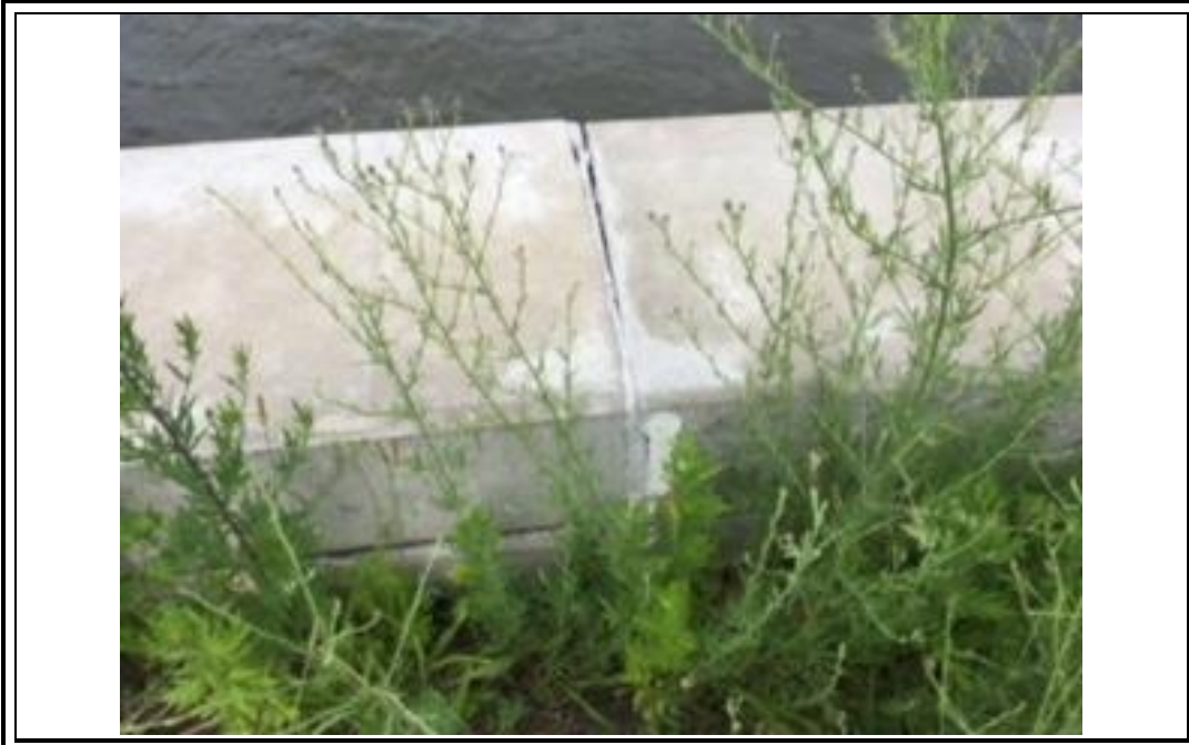
Photograph 9. Significant gap in the precast concrete cap on top of the bulkhead that is angled toward the river. This is consistent with previous site inspections.
