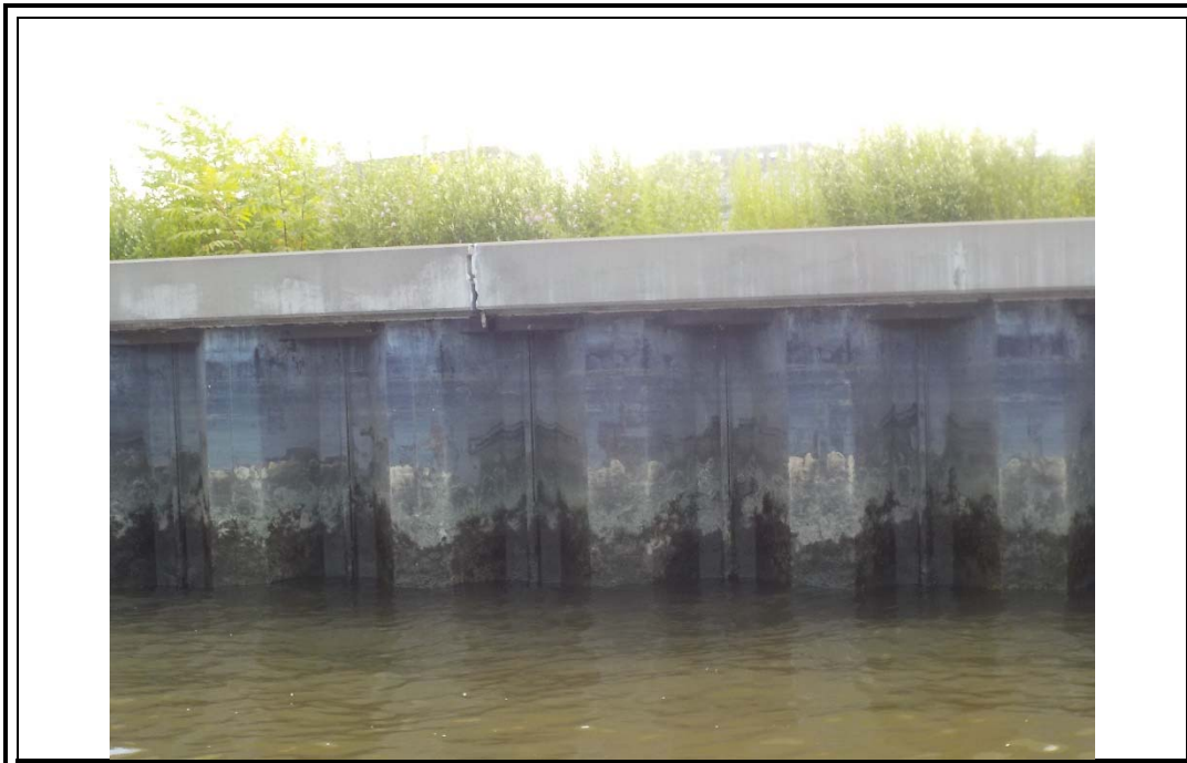
Photograph 10. Crack at a joint in the precast concrete caps on top of the bulkhead.
