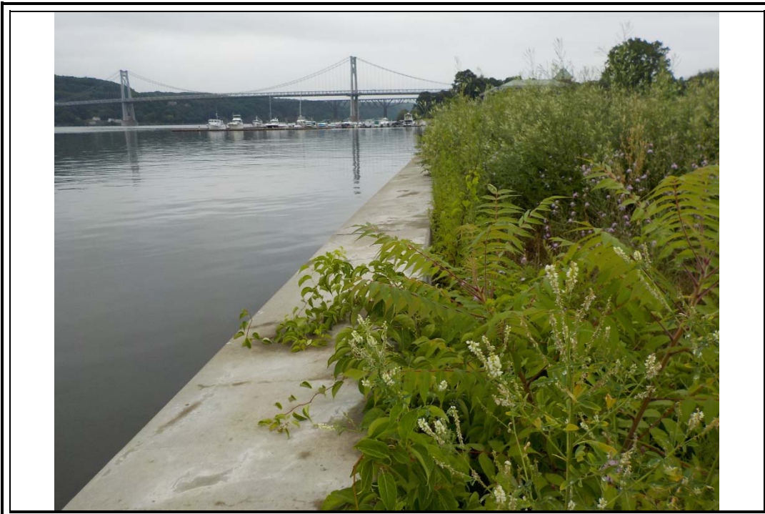
Photograph 6. Slight tilting of bulkhead cap.
