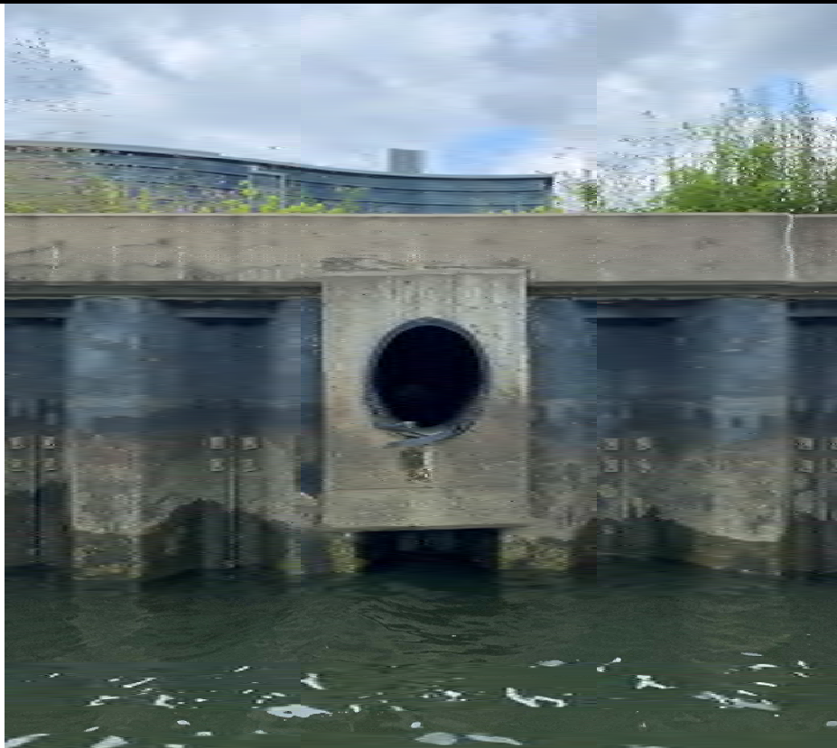
Photograph 8. Storm drainpipe discharging to the Hudson River.
