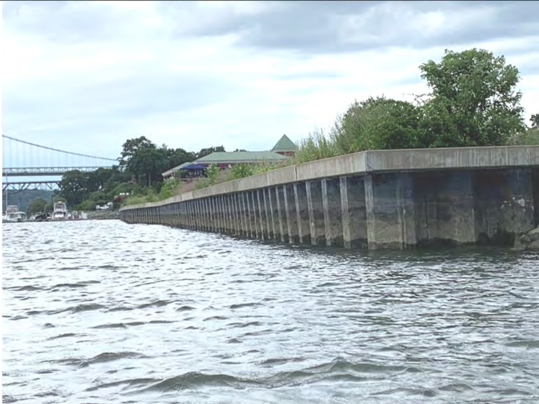
Photograph 10. Zone 3 Bulkhead appears to be leaning toward the Hudson River.
