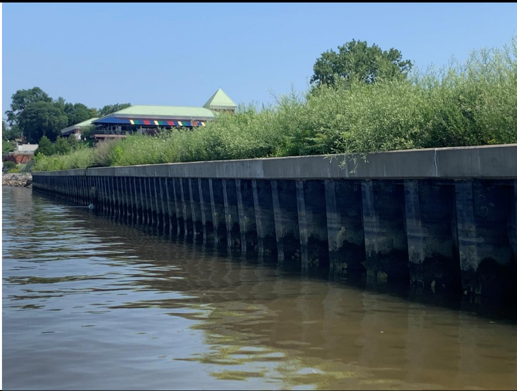
Photograph 9. Zone 3 Bulkhead appears to be leaning toward the Hudson River.
