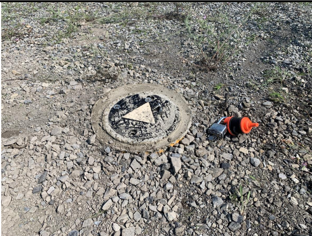
Photograph 13. Permanent flushmount well casing, j-plug, and well lock installed at one out of nine monitoring wells. All monitoring wells enhanced with permanent flushmount casings.
