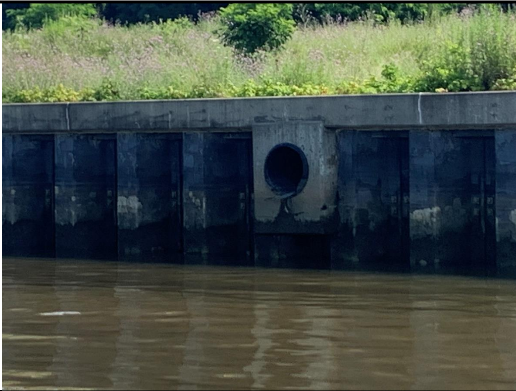
Photograph 7. Storm drainpipe discharging to the Hudson River.
