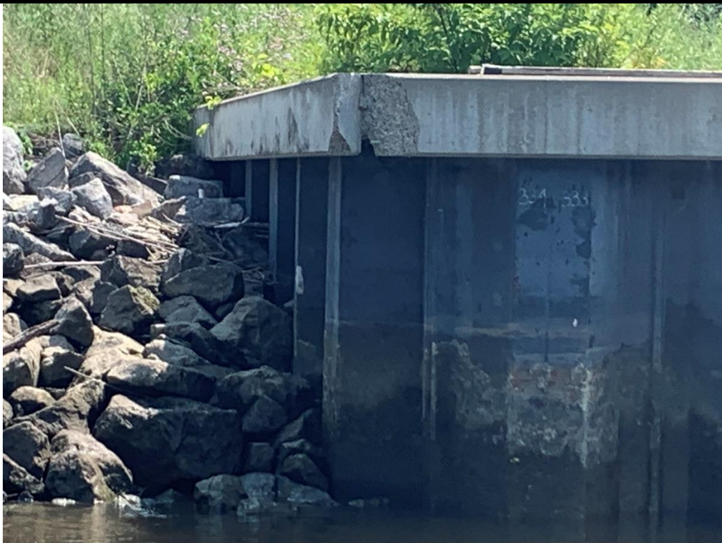
Photograph 11. Separation of precast caps on bulkhead on the far north of the subject site.
