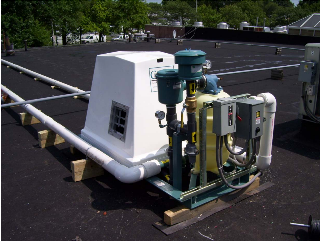
Photograph 10: SVE System after installation
