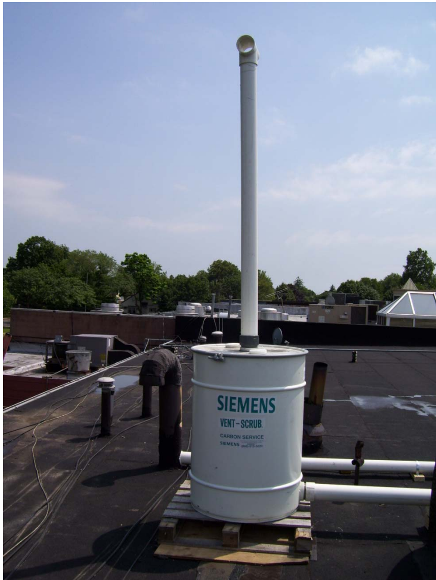
Photograph 12: Vapor-phase carbon-drum on skid.
