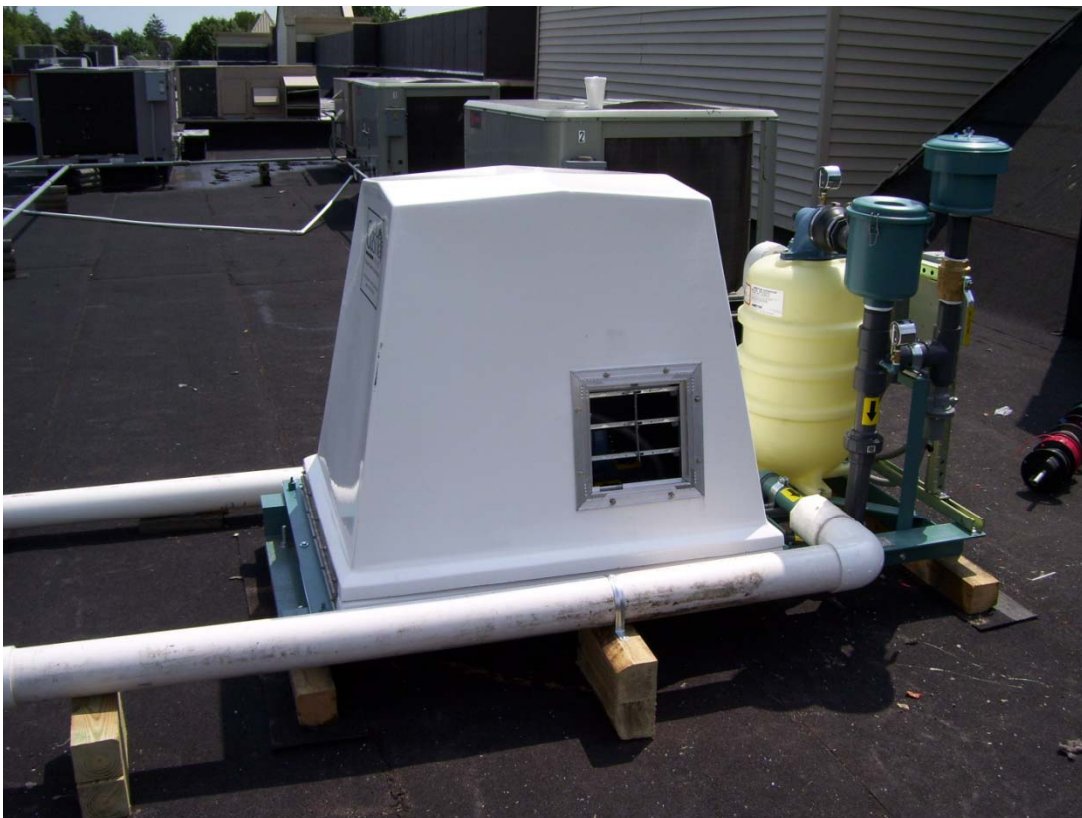
Photograph 7: SVE System after installation.
