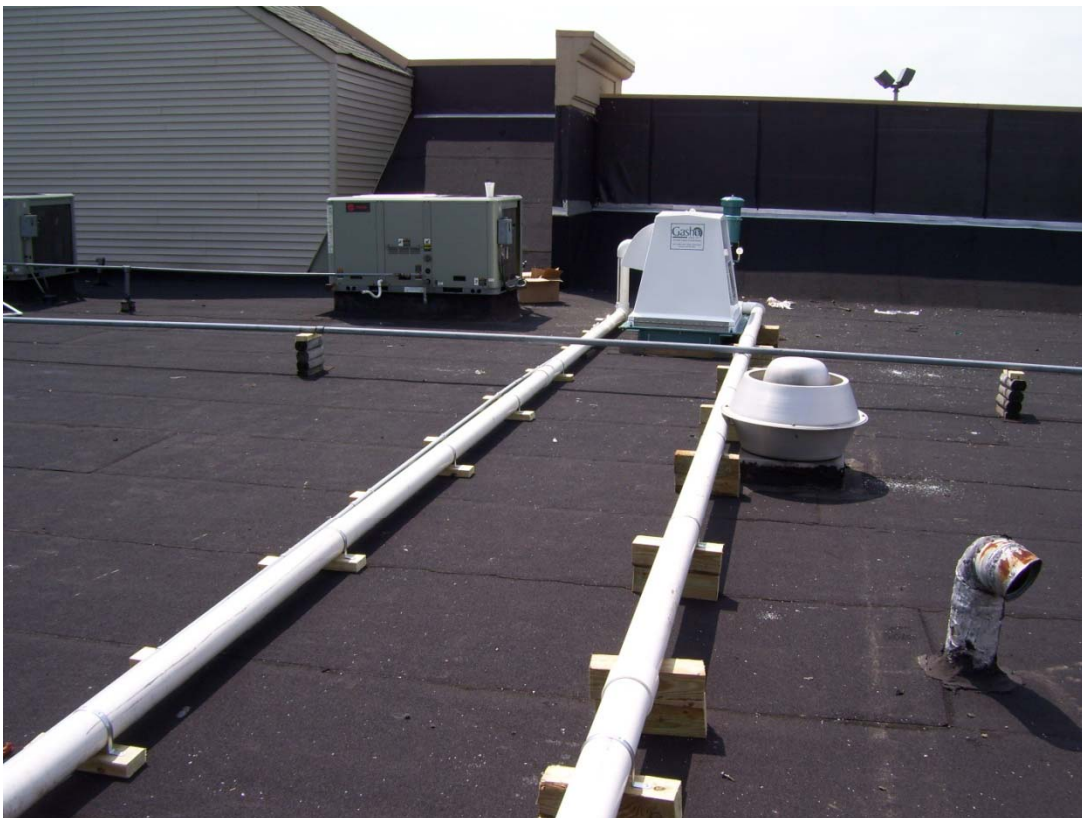
Photograph 9: SVE influent and effluent piping.
