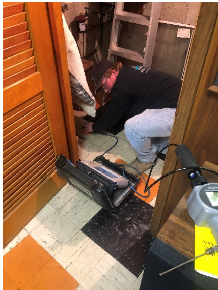
Photo #7: Utility markout prior to sub-slab sample probe installation at 5 University Place
