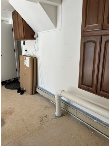
Interior SSD-1 system configuration in garage.
