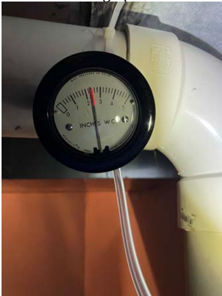
SSD-1 Pressure gauge
