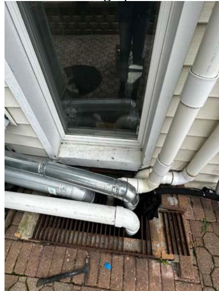
System configuration from the basement window pit
